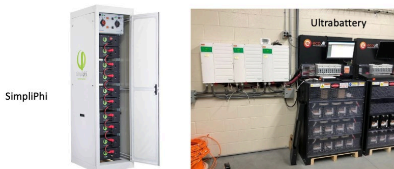
Figure 6. SimpliPhi lithium battery stack, UltraBattery advanced lead-acid stack
