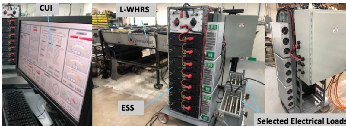
Figure 21. Full-scale operational L-WHRS coupled to ESS “Integration Tower”
