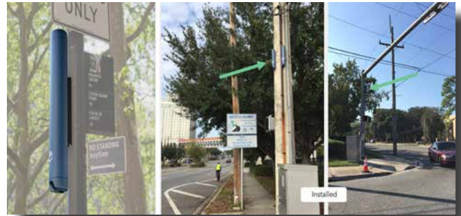
Figure 1 Numina device on a light pole
