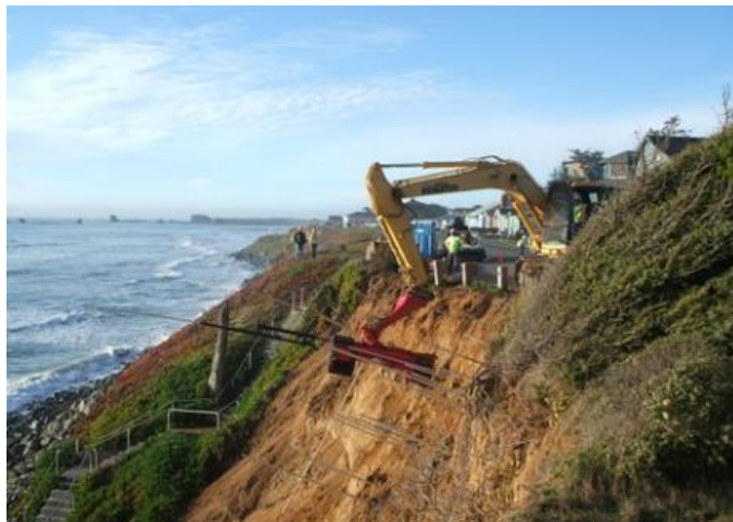
Figure 2. Launched Soil Nails at Pebble Beach Dr., Crescent City, CA (Landslide Solutions, Inc. 2017)
