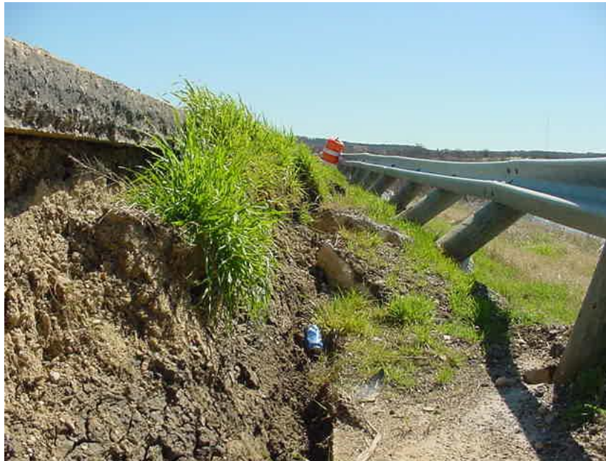
Figure 25. Slope Failure Scarp at Roadway's Edge - Lake Ridge Parkway (Gregory 2006)
