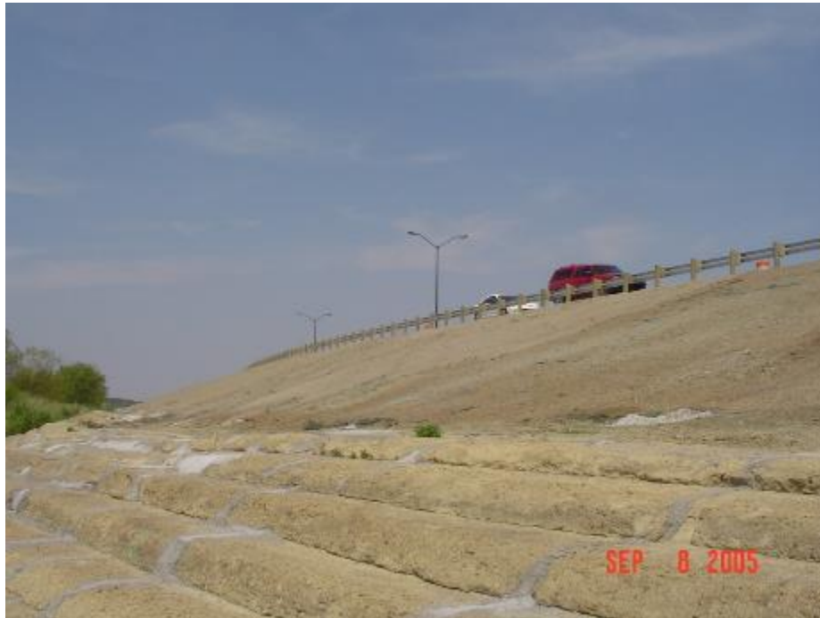
Figure 30. Up-Slope View of Completed FRS Slope Prior to Grass Establishment (Existing Soil-Cement in Foreground) - Lake Ridge Parkway (Gregory 2006)
