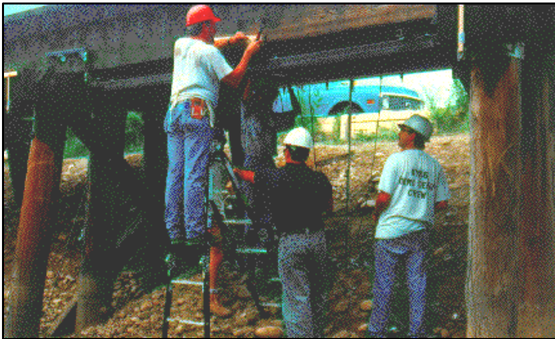
Figure 5-3. Photo of frame for displaced chord instrumentation being installed on Bridge 32.35. Frame is suspended under the bridge chord.
