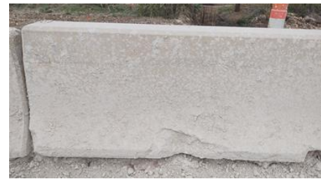
(a) Concrete Spall
