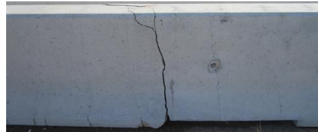
(b) Segment Crack
