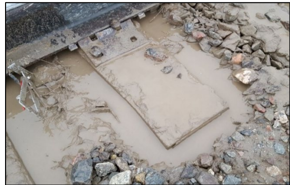
Figure 1. Photograph of mud pumping with standing water
