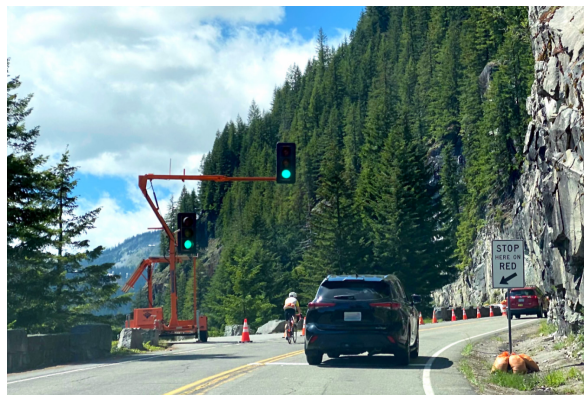
Figure 14. Photo. Temporary signal in Washington. Source: FHWA.
