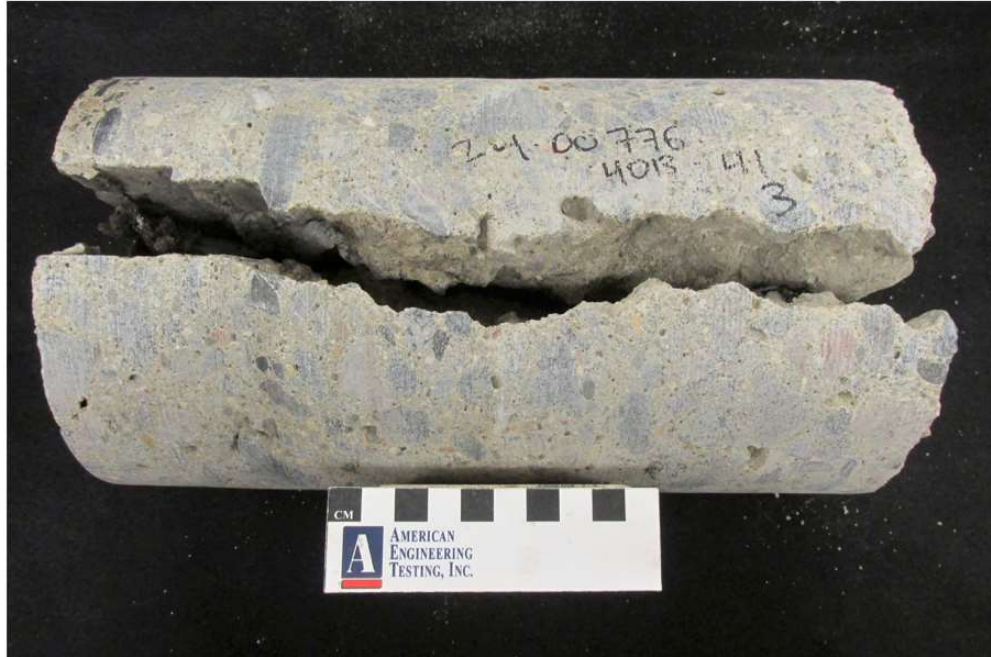
DESCRIPTION – Project 4013-41, core 3
