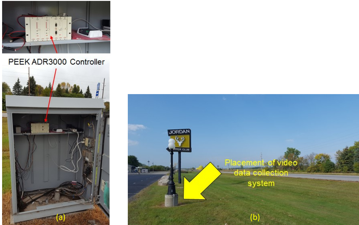
Figure 2.4 PEEK ADR3000 Controller and TIMS Deployment.
