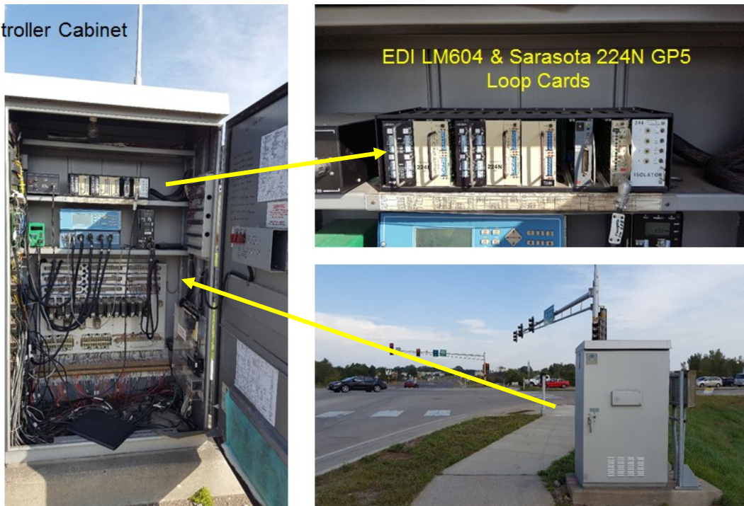
Figure 2.6 Controller Cabinet and Loop Detector Cards at TH169 & TH282 Intersection.
