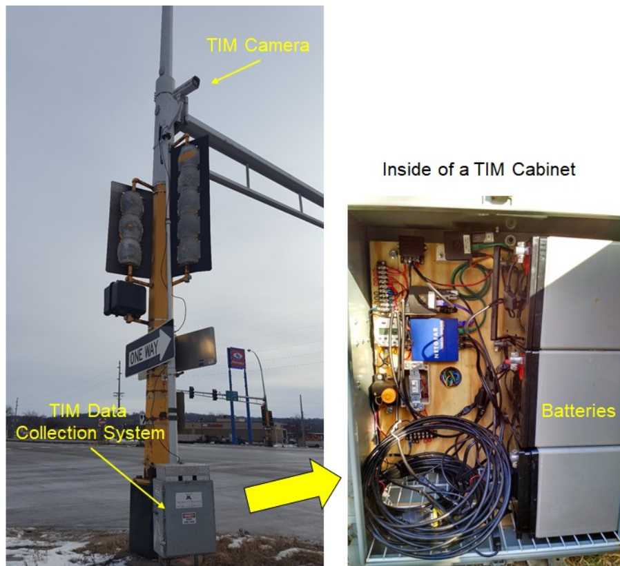
Figure 4.5 TIM Video Data Collection System Installed at Site #2
