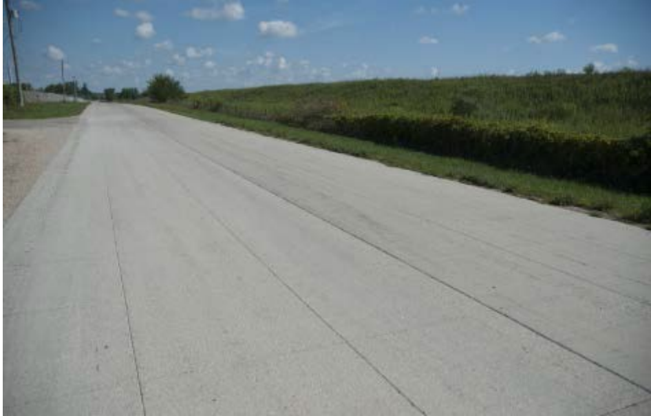
Figure 3-1. Picture of an excellently performing FRC overlay, North Lorang Road, Kane County, IL (King and Roesler, 2014).
