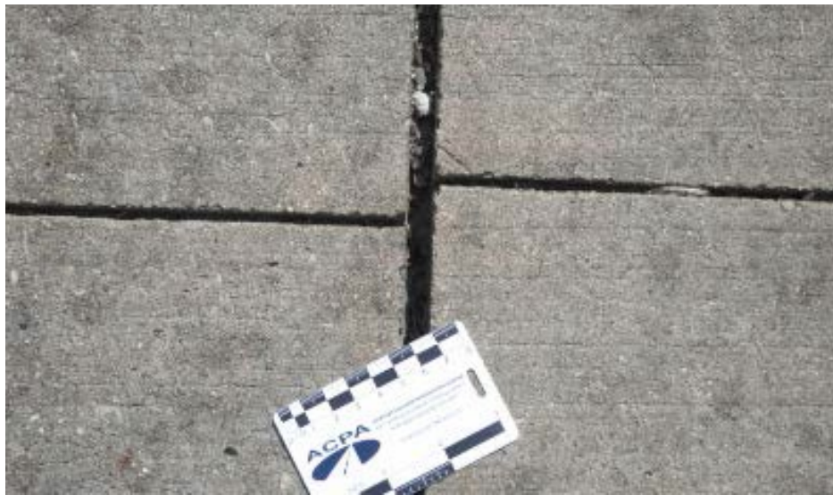
Figure 3-2. Slab migration at the outside longitudinal joint of an overlay project (no fiber) in Illinois (Schank Avenue, Mundelein: (King and Roesler, 2014))
