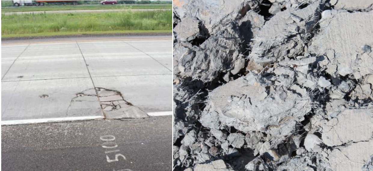
Figure 3-5. (a) Localized distress in Cell 162, (b) fiber visible during removal of distressed concrete (Burnham and Andersen, 2015).
