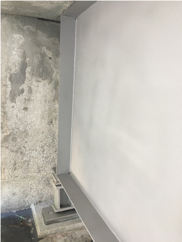
Figure 25 North End of Bridge 40 Hours After Initial Blast
