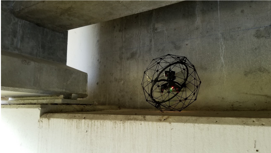
Figure 3.7 Photograph of the Elios UAS Rolling on Top of an Abutment Bearing Seat.
