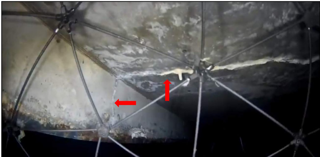
Image 9: Image Clipped from Elios Inspection Video. Inspection of Deck Soffit, note efflorescence and cracking.
