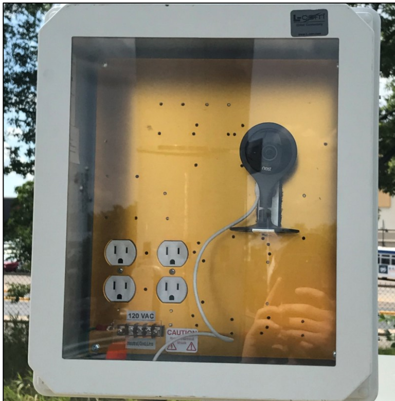
Figure 5-12 - Camera Inside Enclosure
