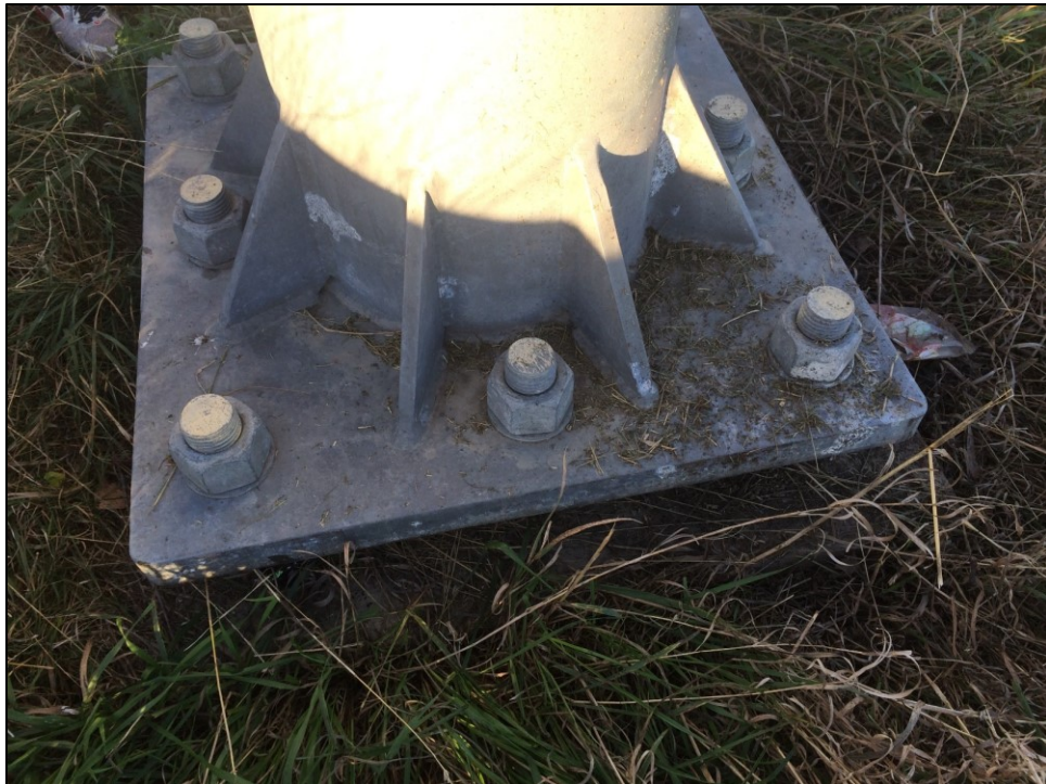
Figure 3-29 - Undersized Washers Found in District 6
