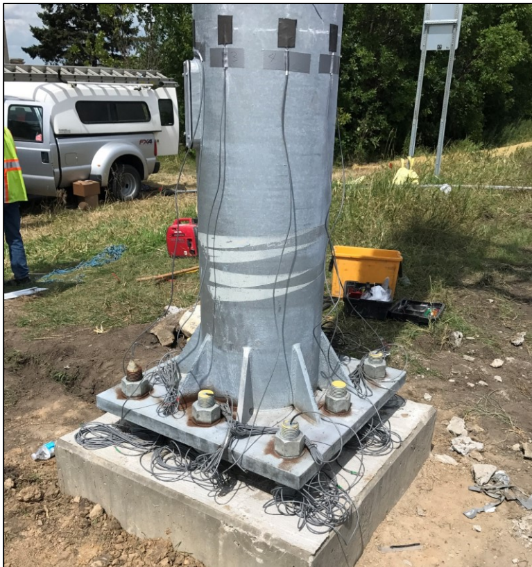
Figure 5-8 - Anchor Bolt and Post Strain Gages
