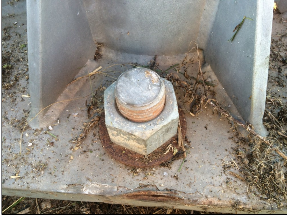
Figure 3-28 - Rusted Washers Found in District 6
