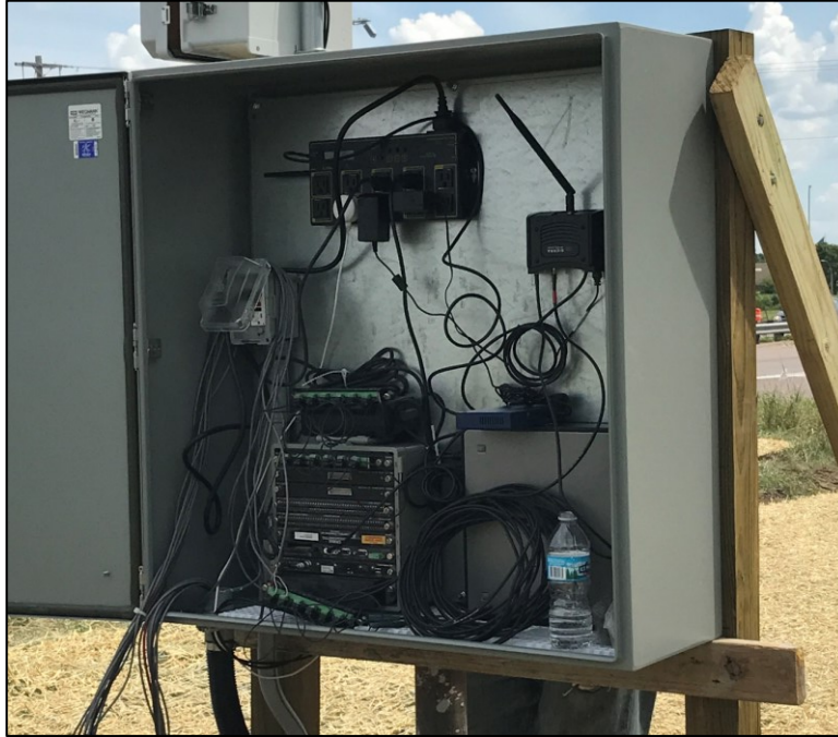
Figure 5-11 - View of Interior of Cabinet
