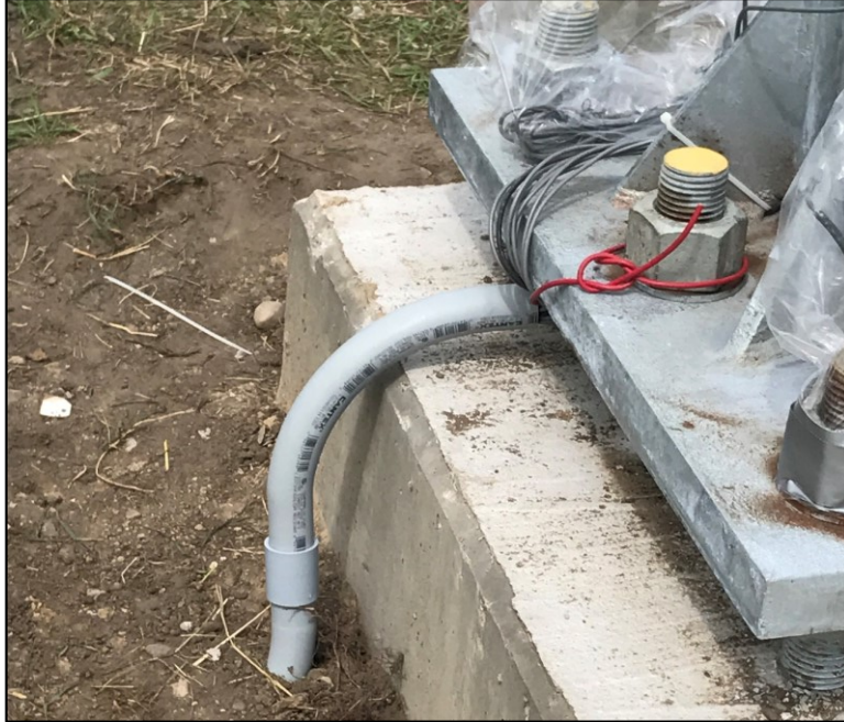
Figure 5-9 - Conduit Leading to Data Logger
