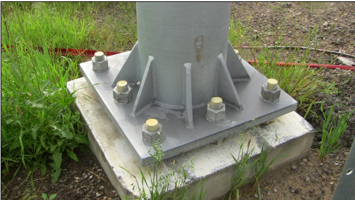
Figure 3-9 - Cantilevered Sign Support Baseplate and Anchor Bolts
