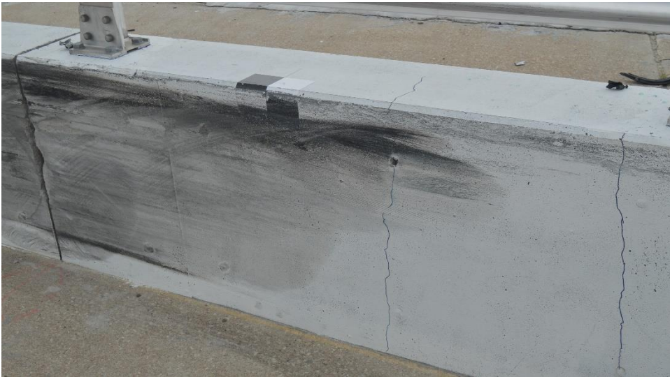
Figure 76. System Damage, Test No. NCBR-2
