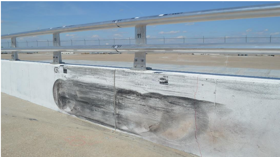
Figure 55. System Damage, Test No. NCBR-1
