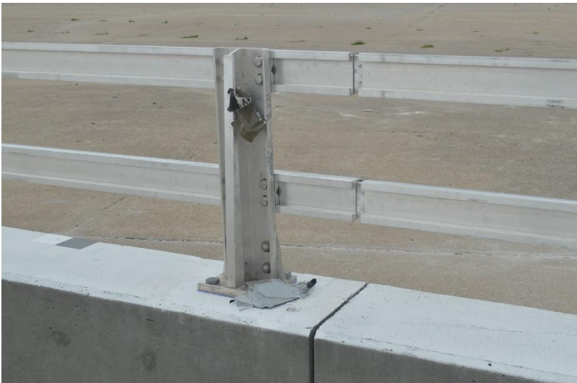
Figure 78. Post No. 6 Backside Damage, Test No. NCBR-2
