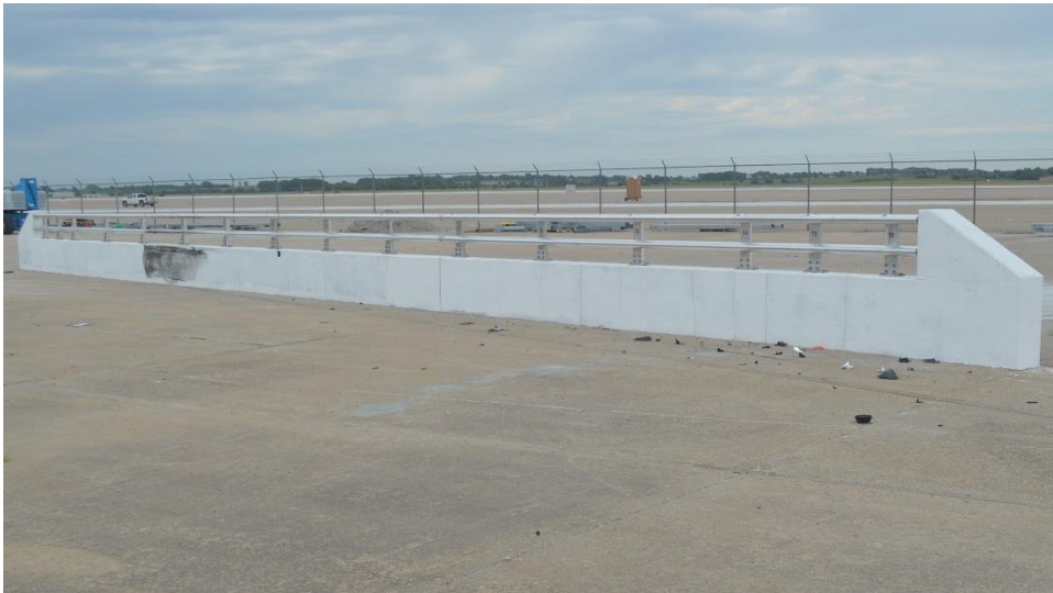
Figure 75. System Damage, Test No. NCBR-2
