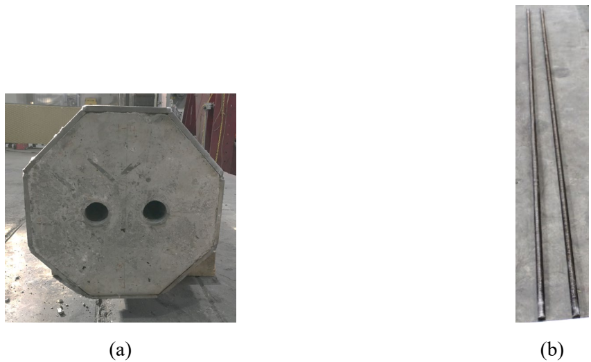
Figure 4.3 Column and PT bar condition after test completion: (a) top of column; (b) PT bars
