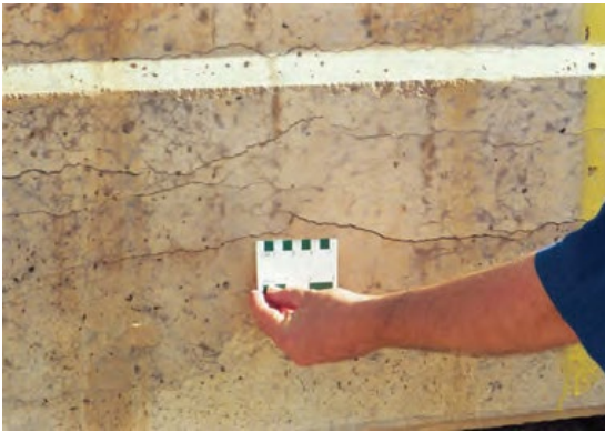
b) PC box beam cracking
