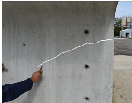
(c) Diagonal cracking – From girder top to girder bottom
