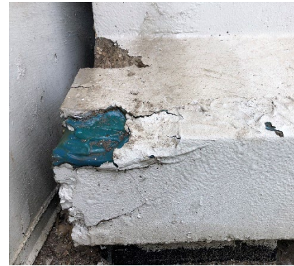
c) Beam end cracking
