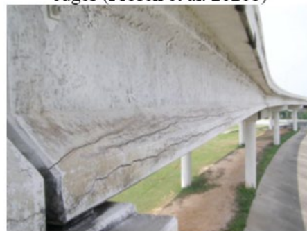
(f) Longitudinal cracks in I-beam bottom flange (Williams and Choudhuri 2010)
