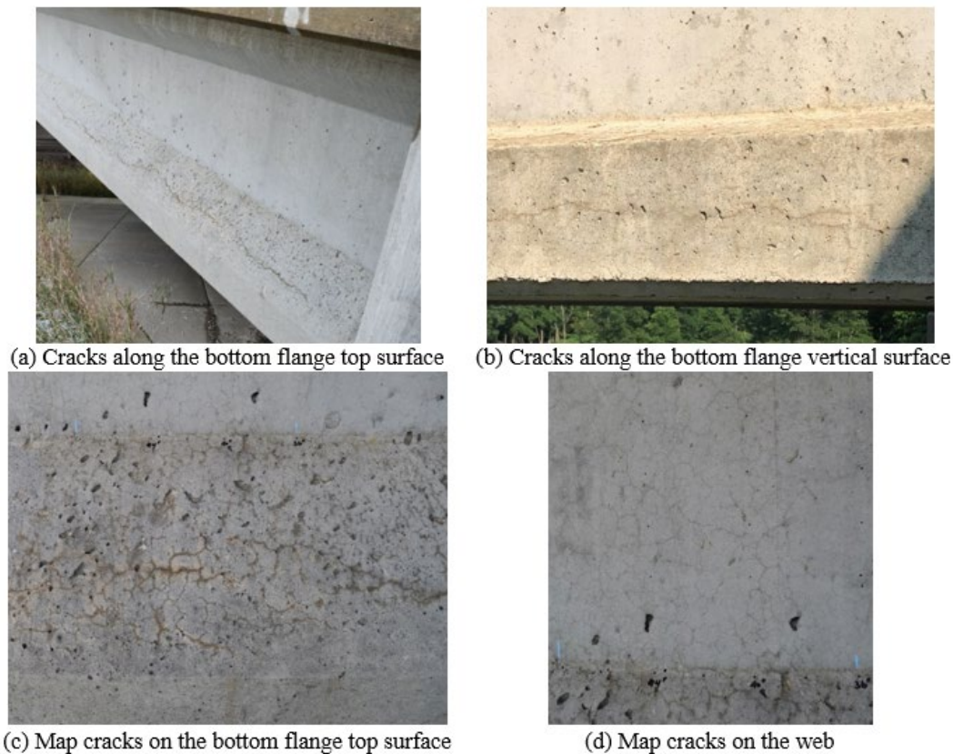
Figure 3-9. Map and longitudinal cracks in PSC I-beams
