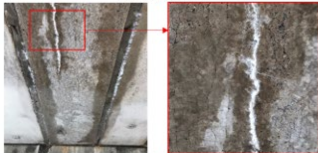
(e) Heavy random cracking (Cracking-PSC 1110) Condition State 4
