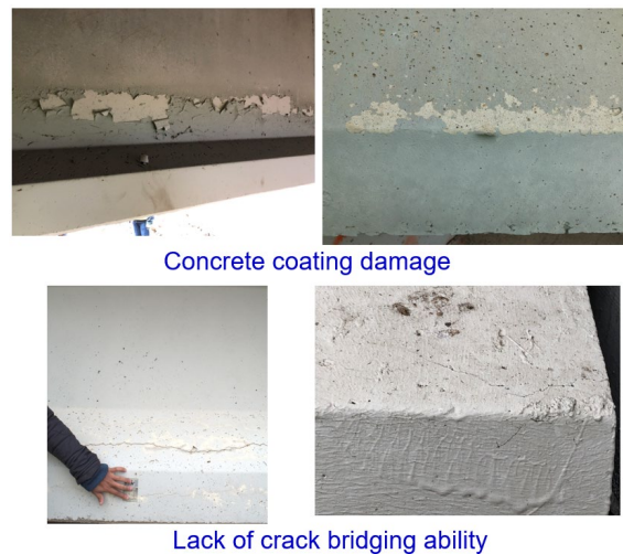
Figure 3-12. Concrete surface coating damage and lack of crack bridging ability
