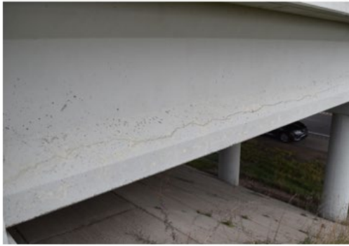
(a) Bottom flange longitudinal cracking
