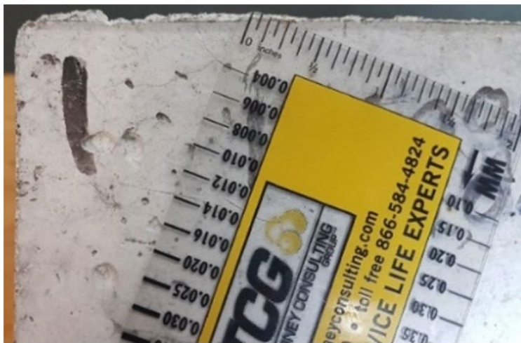
(b) A close-up view showing a 0.004 in. wide crack
