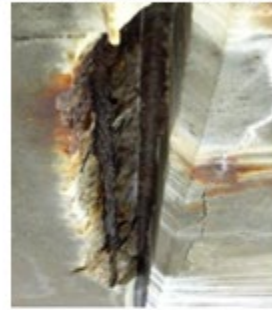
(c) Exposed prestressing with section loss (Exposed Prestressing 1100) Condition State 4
