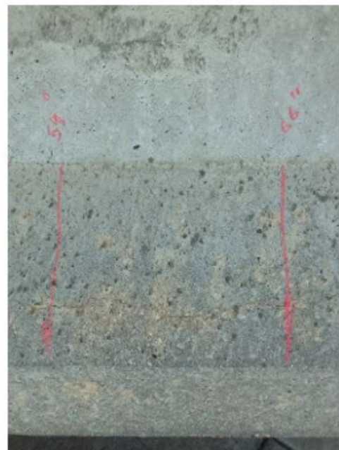
(c) Outside surface of the bottom flange
