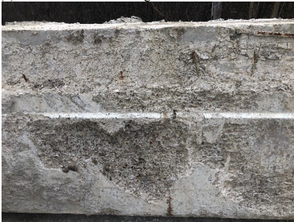
(c) Scaling on the web within beam span
