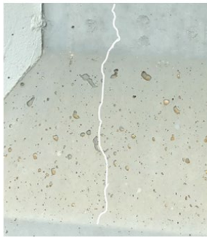
(a) Vertical cracking
