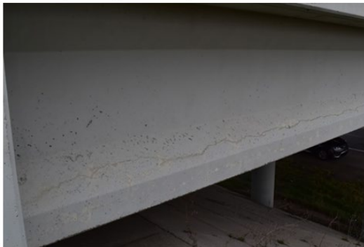
(c) Wide longitudinal cracking (Cracking-PSC 1110), Condition State 3
