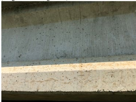
(c) Bottom flange showing longitudinal cracks
