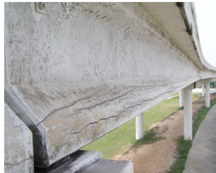
(d) Wide longitudinal cracking (Cracking-PSC 1110), Condition State 4 (Williams and Choudhuri 2010)
