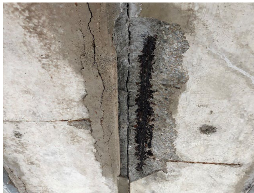
(c) A close-up view of a deteriorated beam
