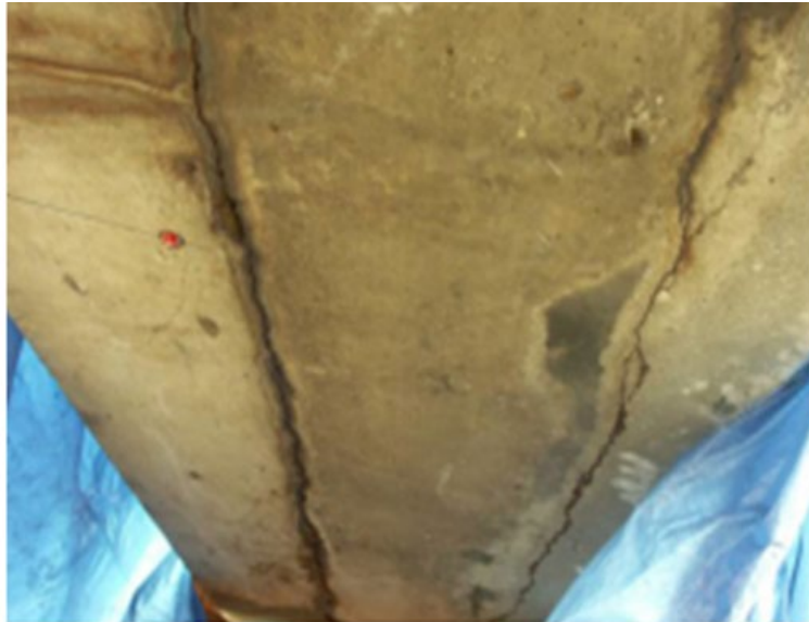
(a) Longitudinal cracking
