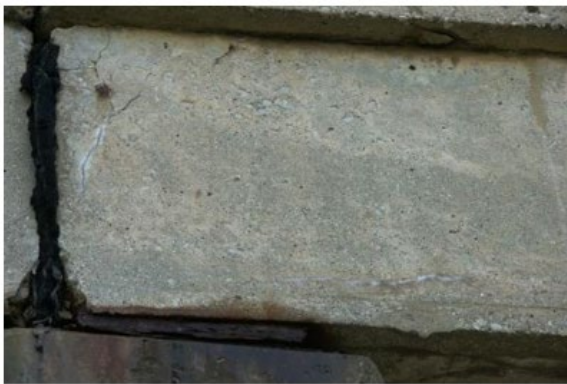
(a) End cracking
