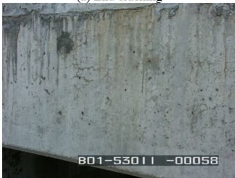
(c) Map cracking on exterior girder web
