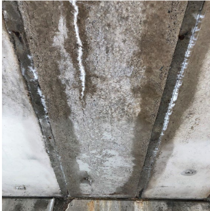
(a) Severe random cracking at beam soffit at beam end
