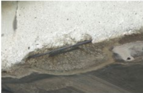
(b) Exposed prestressing with moderate spall (Exposed Prestressing 1100) Condition State 3
