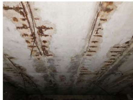
(b) Spalling, corrosion, and broken prestressing strands in box-beams (Frosch et al. 2020a)
