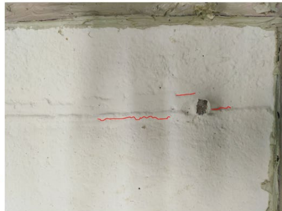
(b) Cracks in Si-Rex 03 applied slabs after 16 days of exposure to 120° F. Red color line represents the cracks in the coating.
