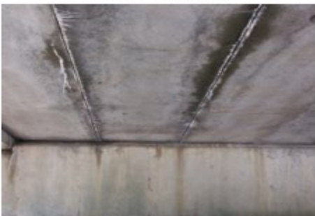
(f) Leaching without rust staining (Efflorescence / Rust Staining 1120) Condition State 2
