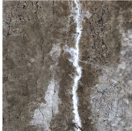
(b) Close up view random cracking at beam end
