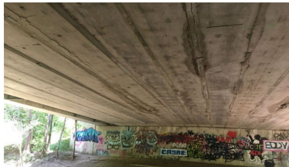
(b) Moist shear keys and longitudinal cracking
