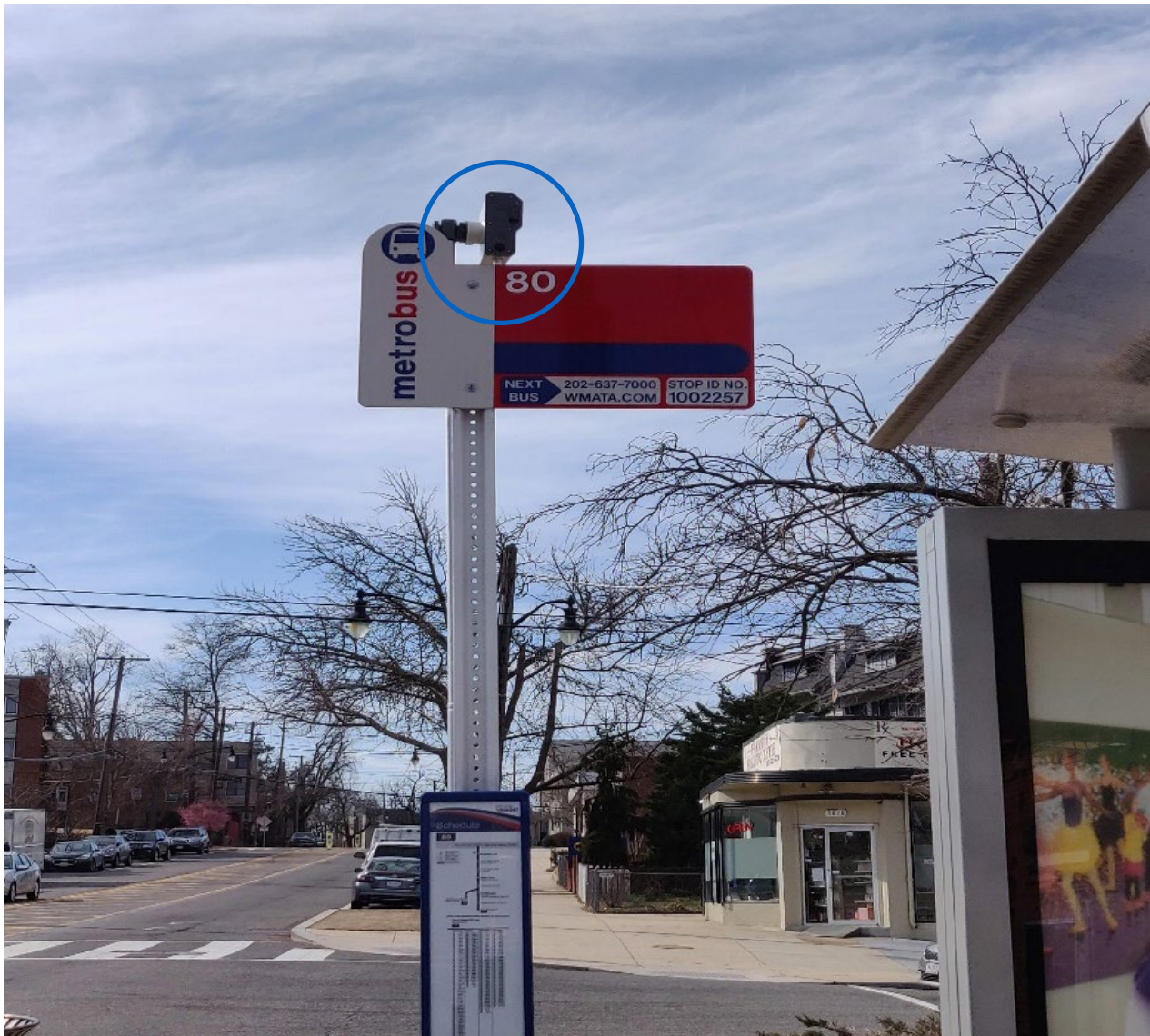
Figure 9. Video Camera Installed at a Selected Bus Stop
