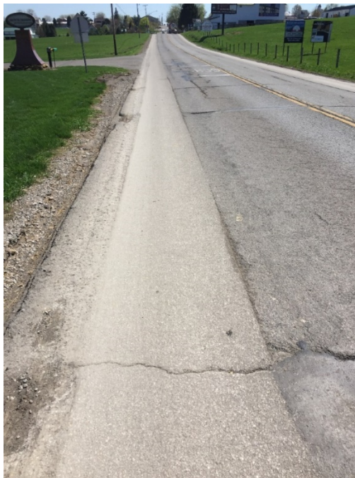
Figure A.9 Pictures of section with AP2-70 mix after 20 months of construction
