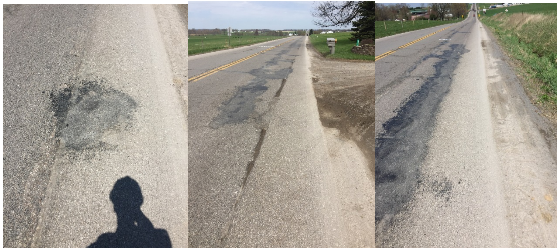
Figure A.11 Pictures of sections with AP2-88 mix after 20 months of construction
