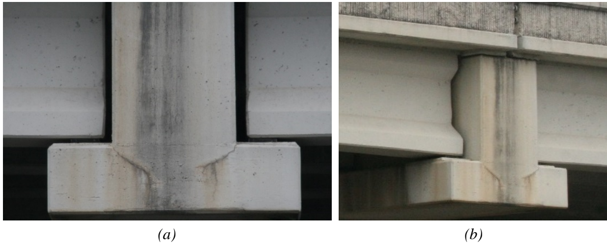
Figure 3.15. Crack at Ledge-Flange Interface of Exterior of Bent 29.
