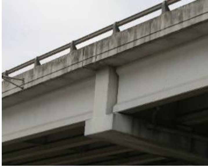
Figure 3.9. Edge of Deck Extends Past End of Inverted-T Bent Caps.
