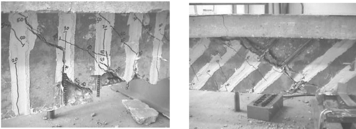
Figure 2.13. Vertically and Diagonally Mounted Near-Surface FRP Rods after Failure (DeLorenzis and Nanni, 2001).
