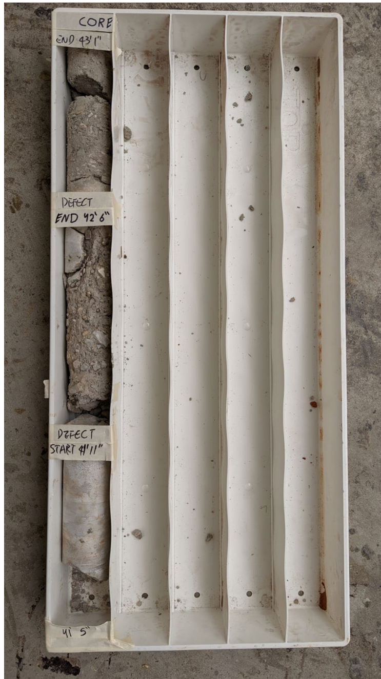
Figure 159. Photo. Photograph showing a core obtained from test shaft #3 showing the start and end of observed defect between a depth of 41 ft 11 in. and 42 ft 6 in from core #2 of test drilled shaft #3.
