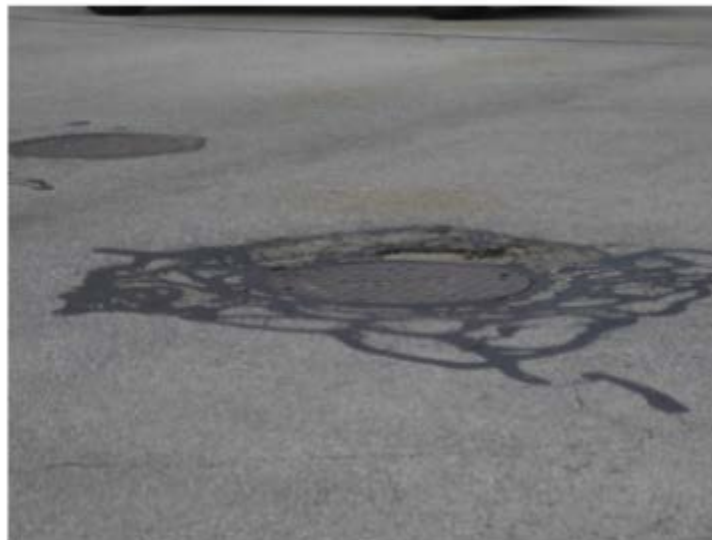
Figure 18. Excess Sealant (Tar Snakes) Reduces Surface Friction (54).
