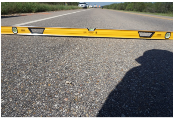
Rutting in Outer Wheel Path: 1/16-8/16 in. 10/09/2017
