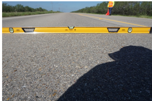
Rutting in Inner Wheel Path: 1/16 in. 10/09/2017
