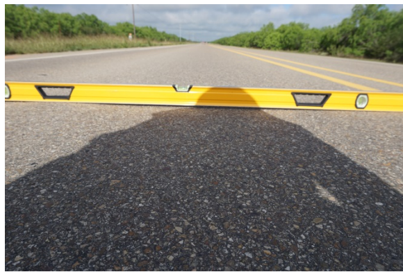
Rutting in Inner Wheel Path: 1/16-8/16 in. 03/29/2018
