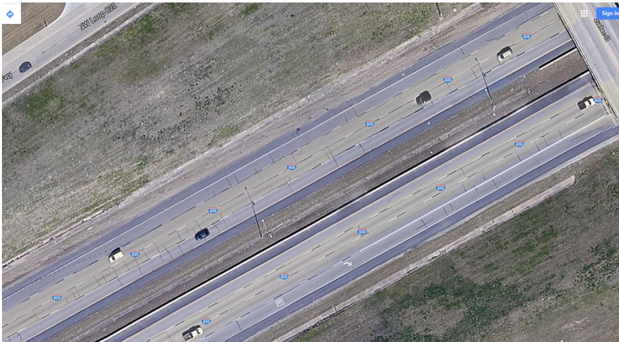
Satellite View Accessed on 06/25/2018 via Google Map Figure 9. Loop 820 Test Sections: Cracking Conditions.
