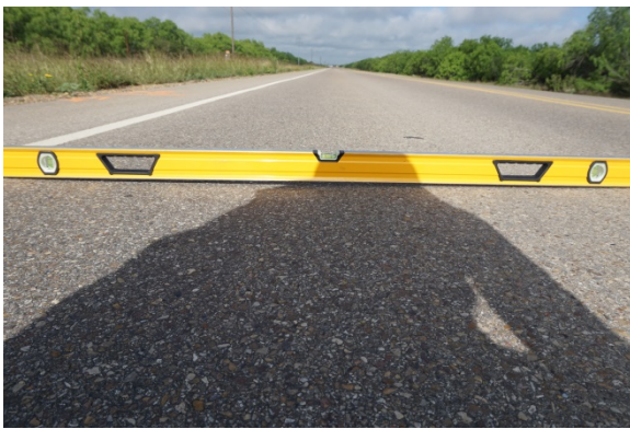
Rutting in Outer Wheel Path: 1/16-8/16 in. 03/29/2018
