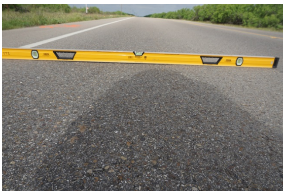
Rutting in Outer Wheel Path: 2/16-3/16 in. 03/29/2018
