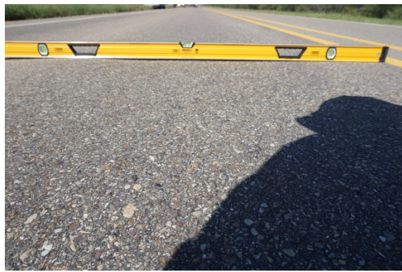
Rutting in Inner Wheel Path: 1/16-8/16 in. 10/09/2017
