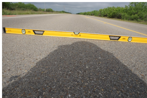
Rutting in Inner Wheel Path: 1/16 in. 03/29/2018
