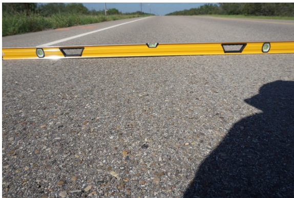
Rutting in Outer Wheel Path: 1/16-2/16 in. 10/09/2017
