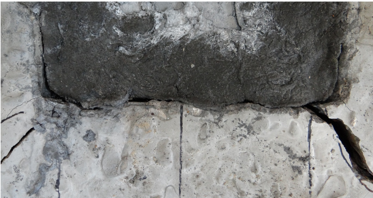
Figure 68. Vertical deformation of the central repair slab and cracks propagating from the corner of the repair slab into the supporting outer slab.
