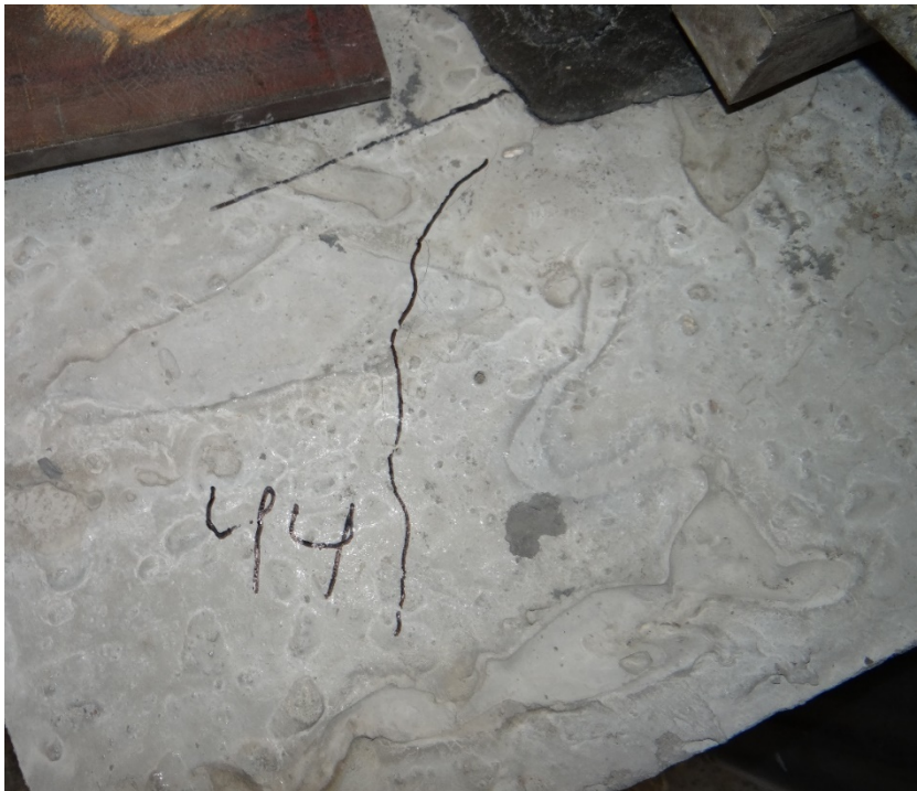
Figure 66. Initiation of cracks from the corner of the repair joint at 44 kips of the post peak vertical load.
