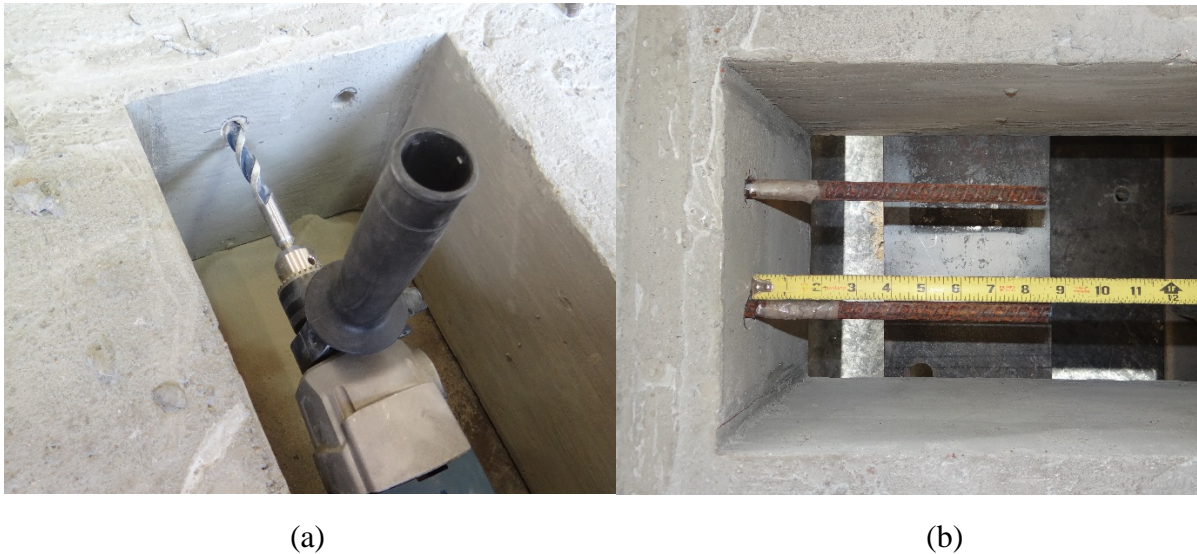
Figure 30. (a) Drilling in the outer hollow slab for rebar placement and (b) rebar length inside the newly repaired concrete.
