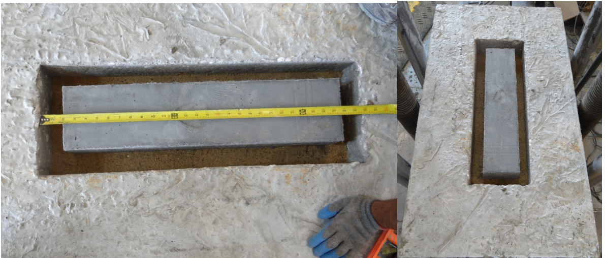
Figure 38. Placement of precast UHP-FRC panel into hollow portion of outer hollow slab.
