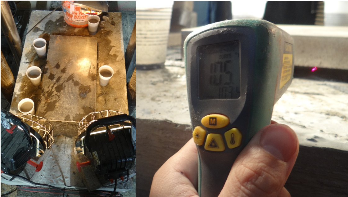
Figure 40. The cast-in-place UHP-FRC repair joint heated to an average temperature of 100 °F using a combination of heaters.
