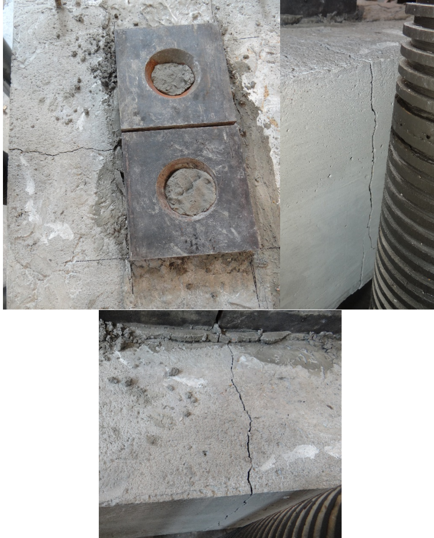
Figure 61. Cracks seen at mid-span of the longer dimension extending throughout the depth of the slab.
