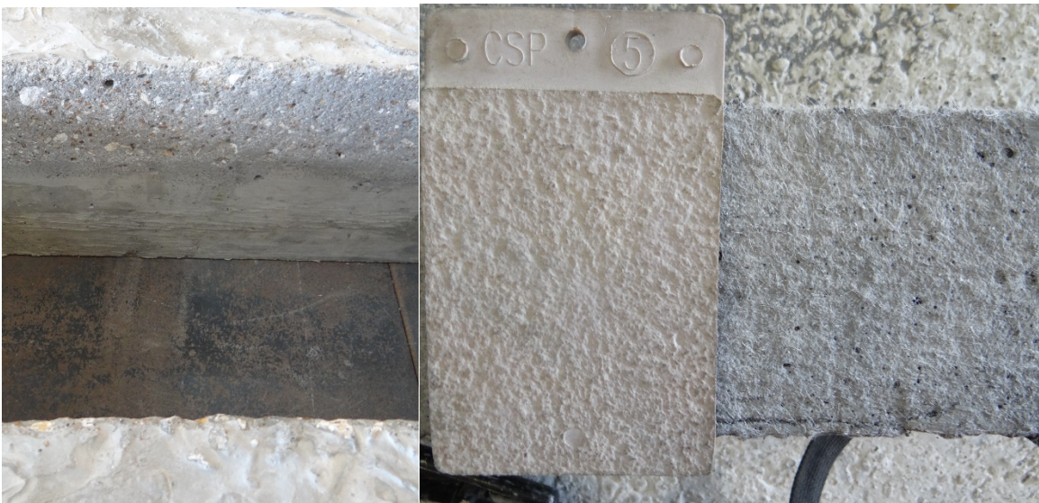
Figure 36. Roughened surface of inner wall of the outer hollow slab with a depth of 4 inches with a roughness level of CSP 5.
