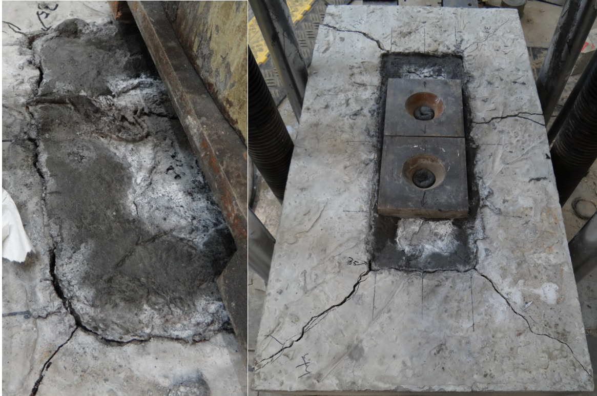
Figure 67. Interface crack caused due to vertical slip and cracks observed on the outer support slab.
