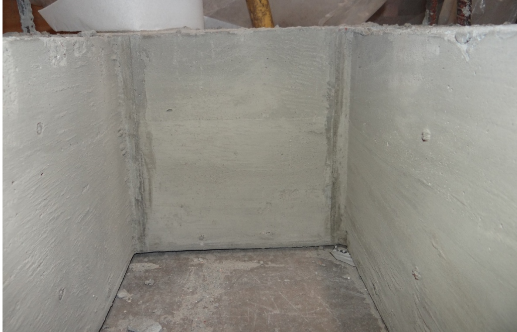
Figure 29. Concrete surface roughness (cast in contact with wood formwork).
