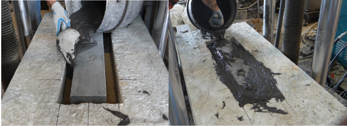
Figure 39. Cast in place UHP-FRC between the precast UHP-FRC slab and outer hollow slab.
