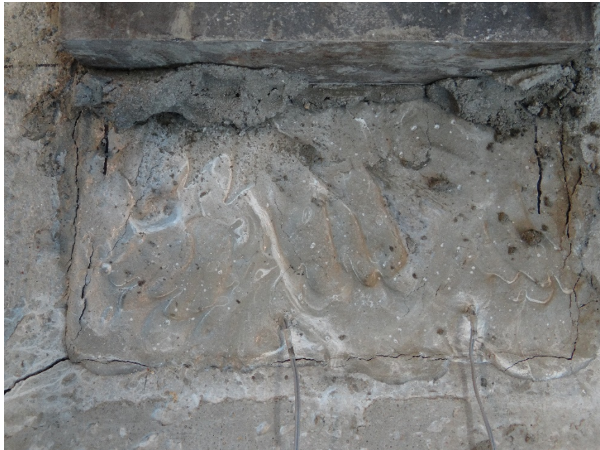
Figure 59. Cracks observed at the interface between repair cast in place PC and the old concrete (outer hollow slab) post peak.
