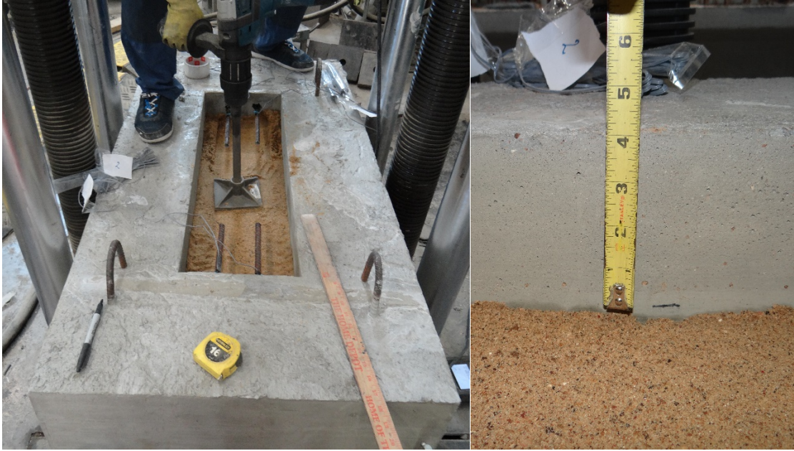
Figure 33. Placing and compacting the sand in the hollow portion of the slab to provide a firm support for casting 4 inches of cast-in-place PC.
