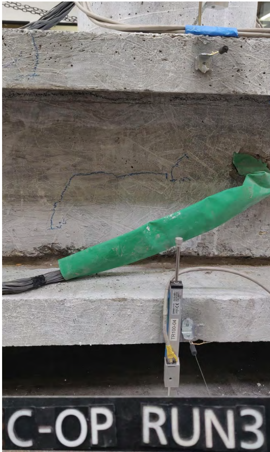
Figure 5.4 Shear and torsion cracks on cap beam south side after run 3
