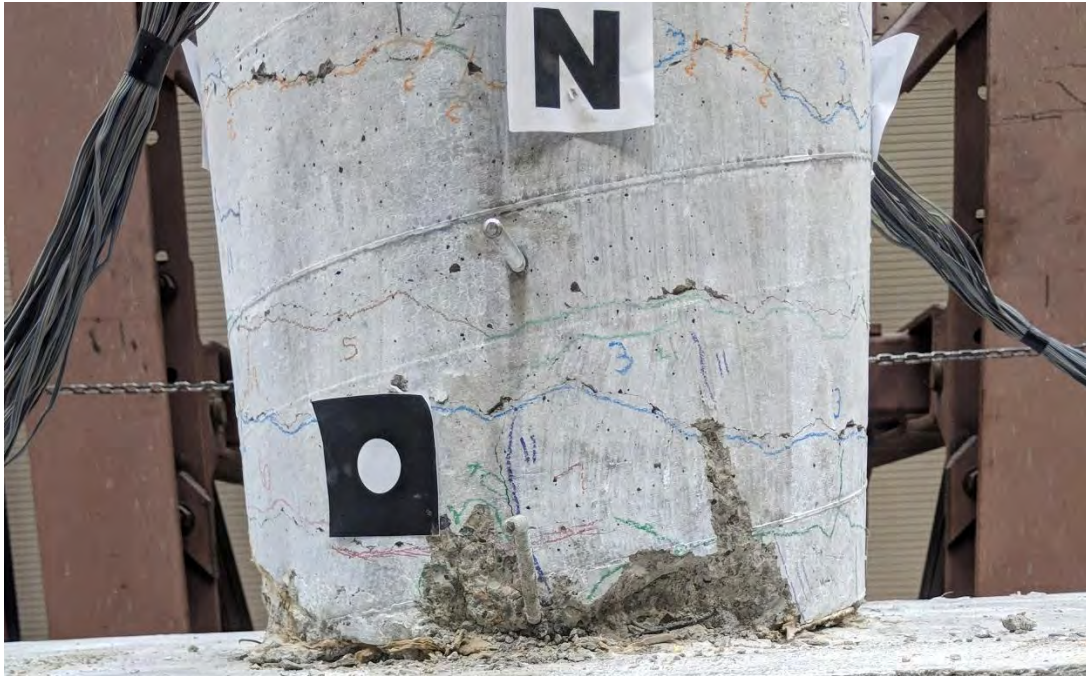
Figure 5.14 Concrete spalling on column north side after run 11 (final run)
