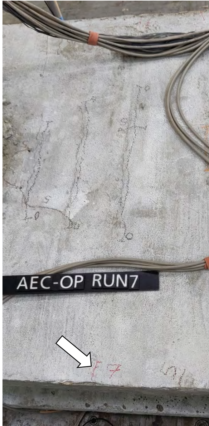
Figure 5.9 Torsion crack in cap beam flange after run 7
