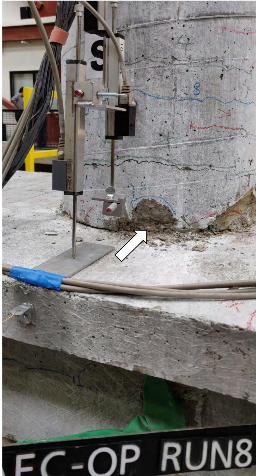
Figure 5.8 Concrete spalling on column south side after run 8
