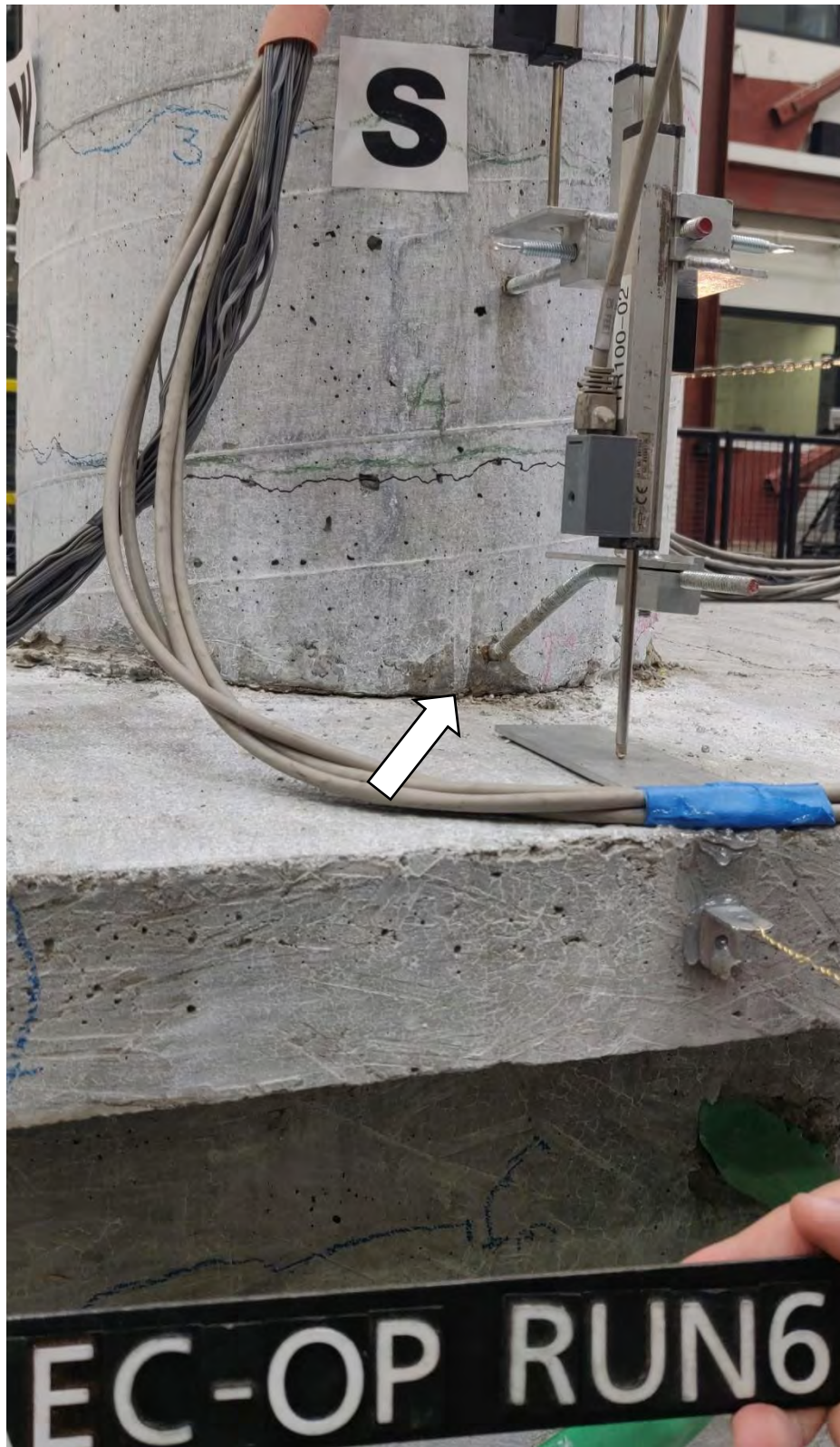
Figure 5.7 Concrete spalling on column south side after run 6
