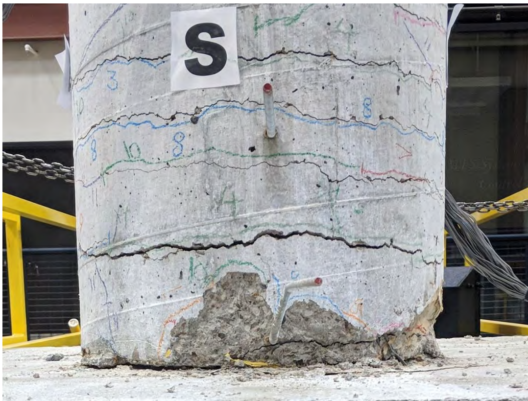
Figure 5.15 Concrete spalling on column south side after run 11 (final run)
