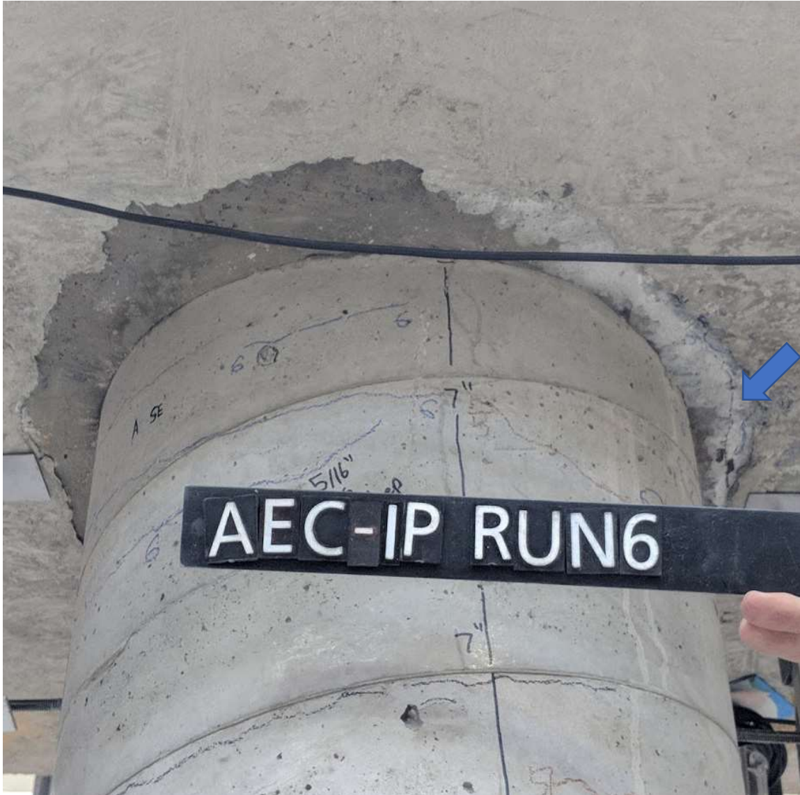
Figure 5.7 Run 6 – Extension of flexural cracks and grout crack (ABC - E face)
