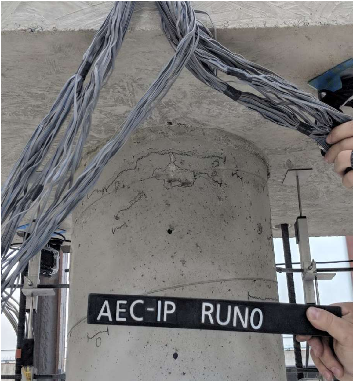
Figure 5.26 Run 0 – Voids marked before testing (CIP – W face)
