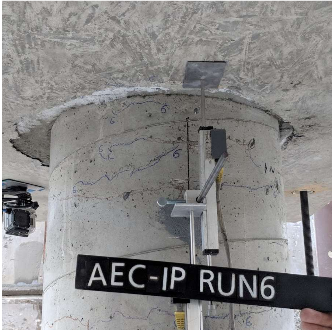
Figure 5.8 Run 6 – Appearance and extension of flexural cracks (ABC - N face)
