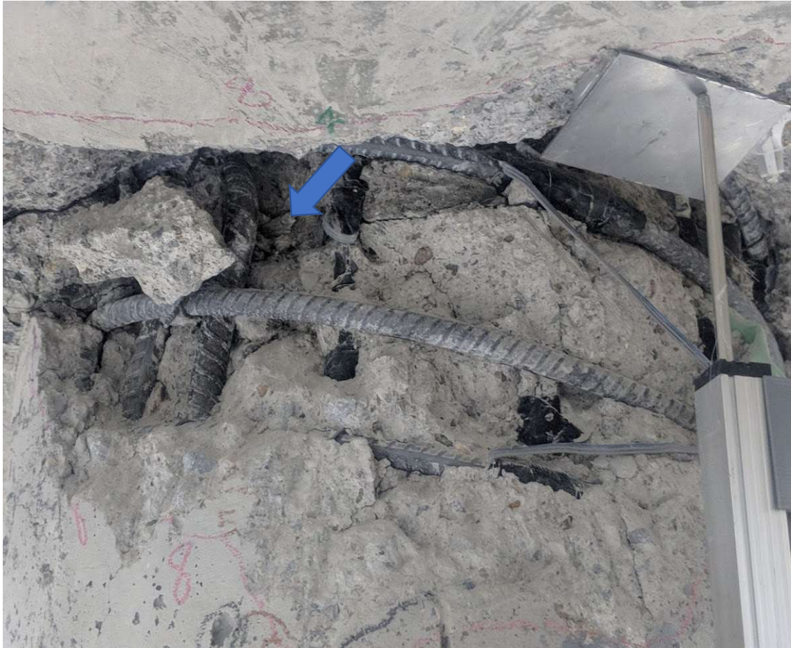
Figure 5.45 Run 9 – Close up of damage on southern face and deformed bars (CIP – S face)
