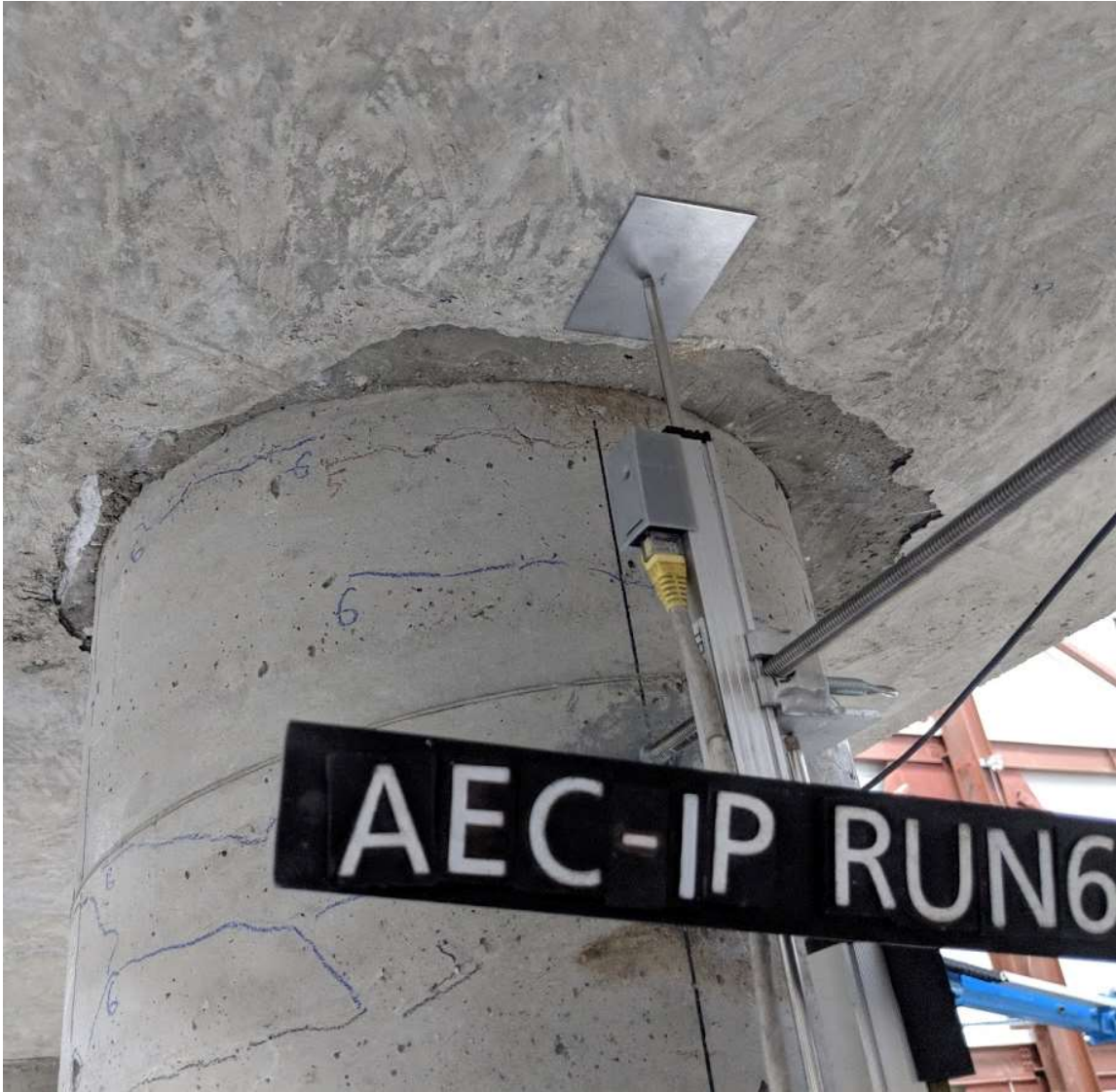
Figure 5.9 Run 6 – Appearance and extension of flexural cracks (ABC - S face)
