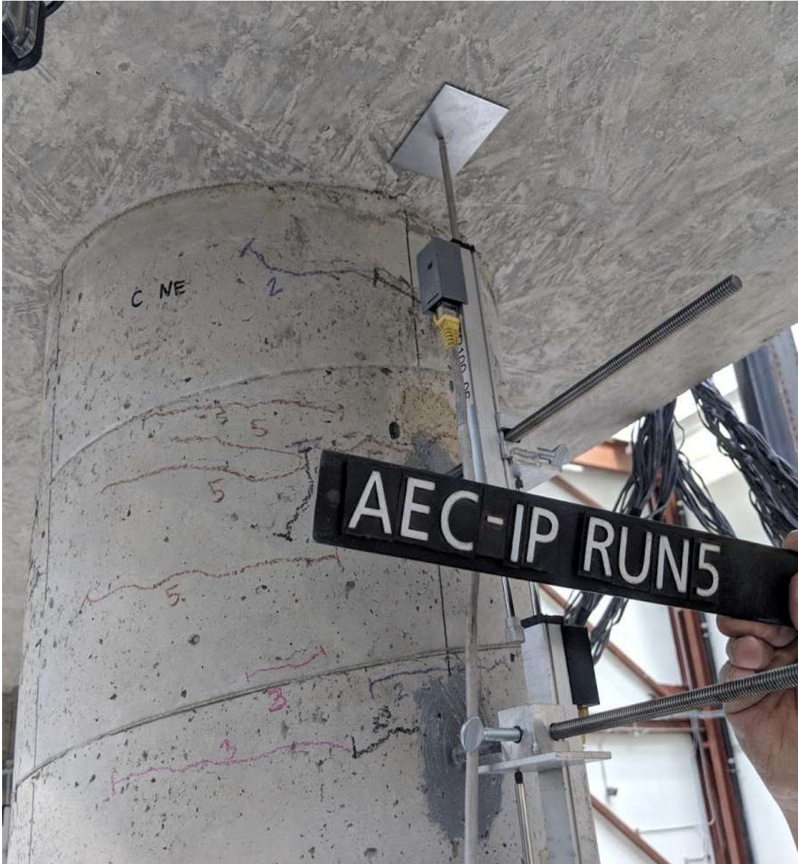
Figure 5.31 Run 5 – Appearance of several flexural cracks (CIP – N face)
