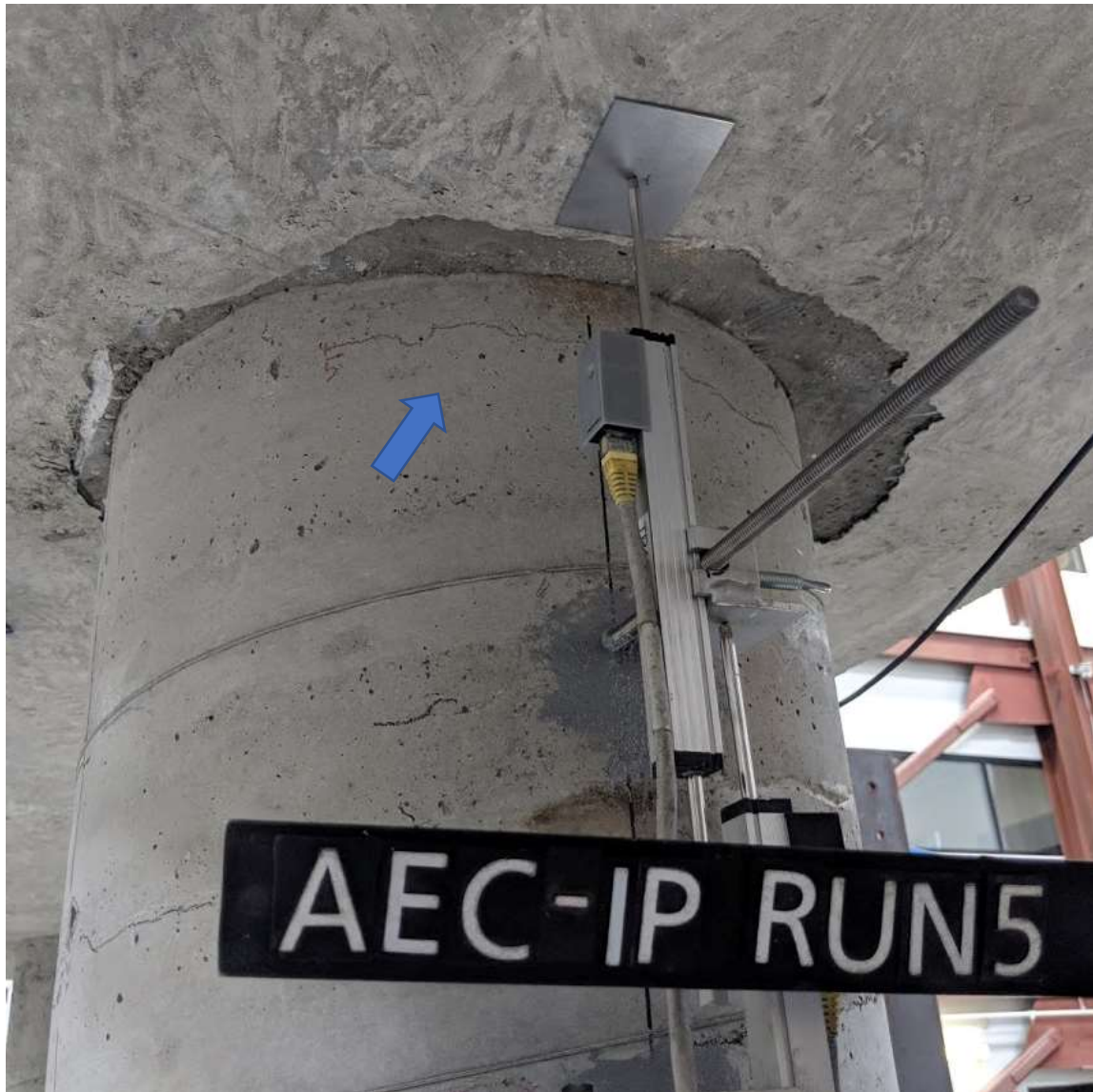
Figure 5.6 Run 5 – Appearance of flexural cracks in plastic hinge (ABC - S face)
