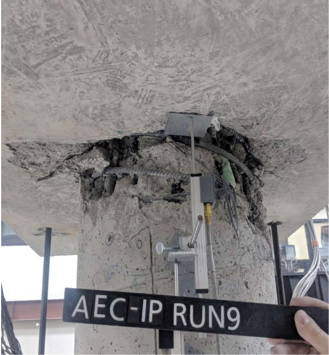
Figure 5.42 Run 9 – Progression of spalling into cap beam and column core (CIP – S face)
