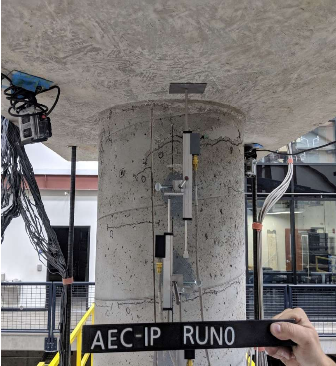
Figure 5.25 Run 0 – Cracks marked before testing (CIP – S face)
