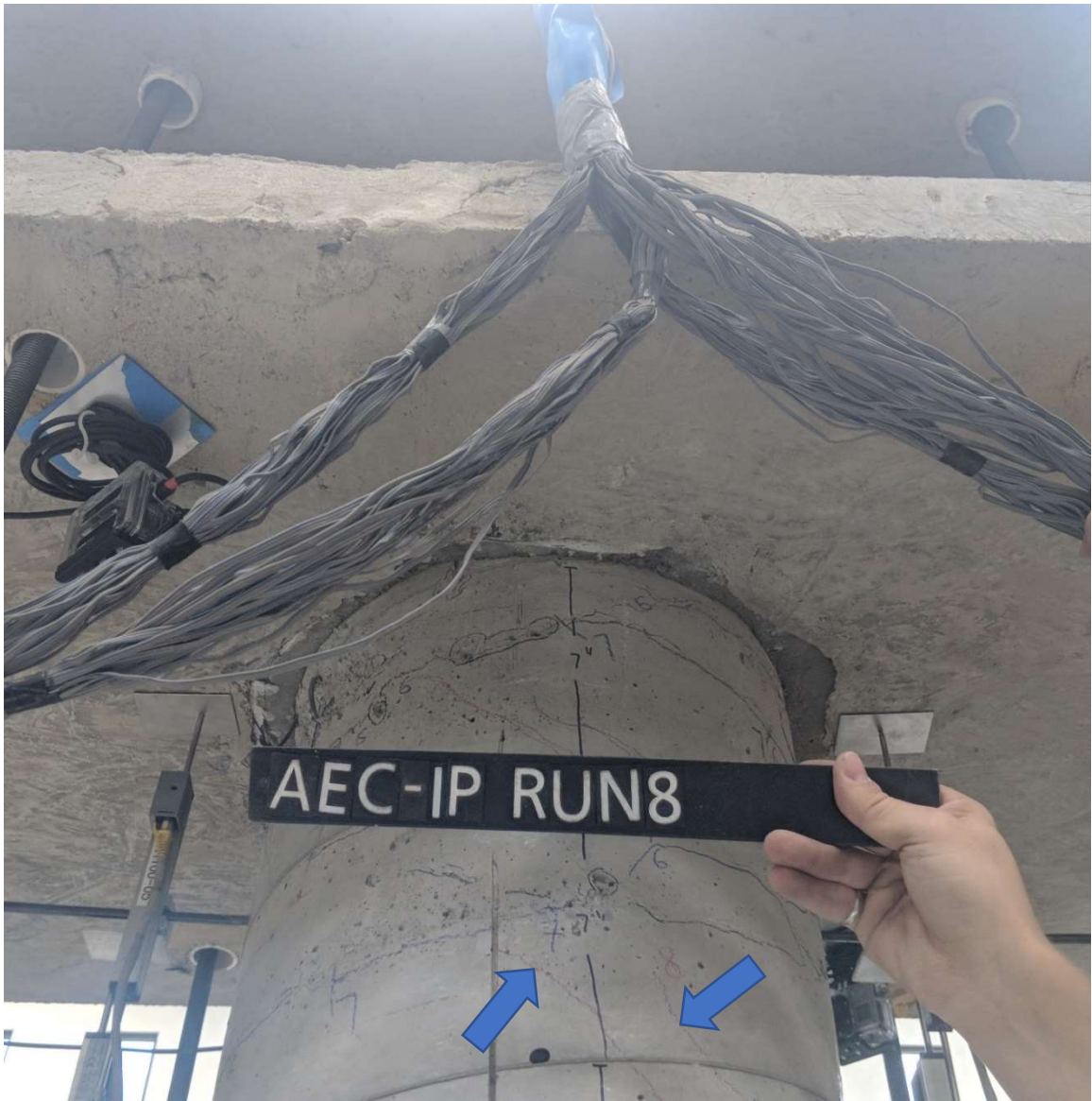
Figure 5.14 Run 8 – Appearance of shear cracks (ABC – W face)
