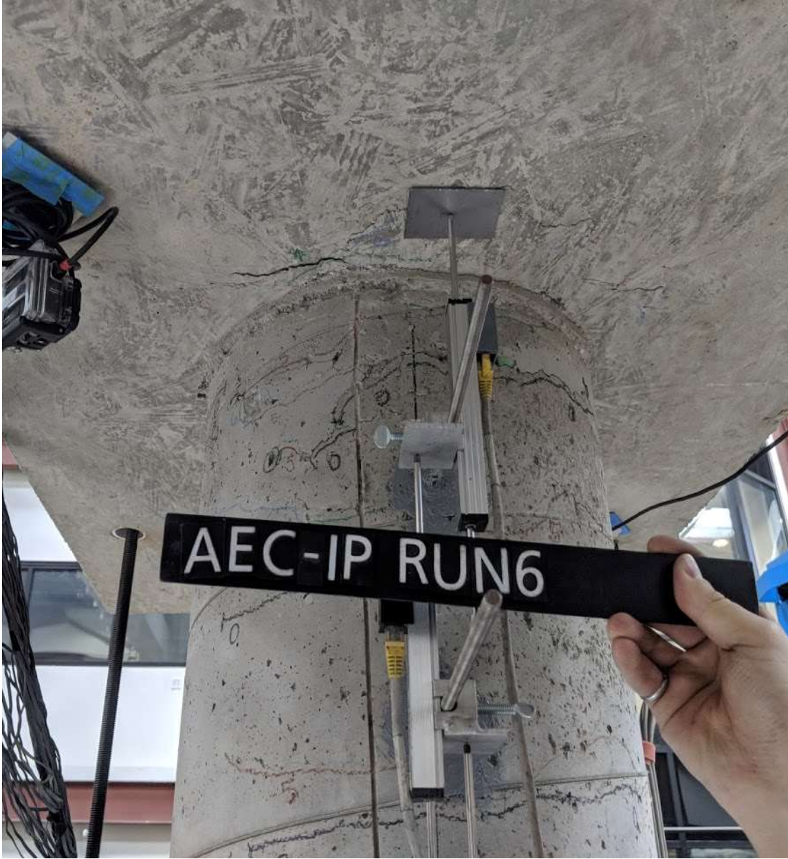
Figure 5.34 Run 6 – Cracks marked before testing (CIP – S face)
