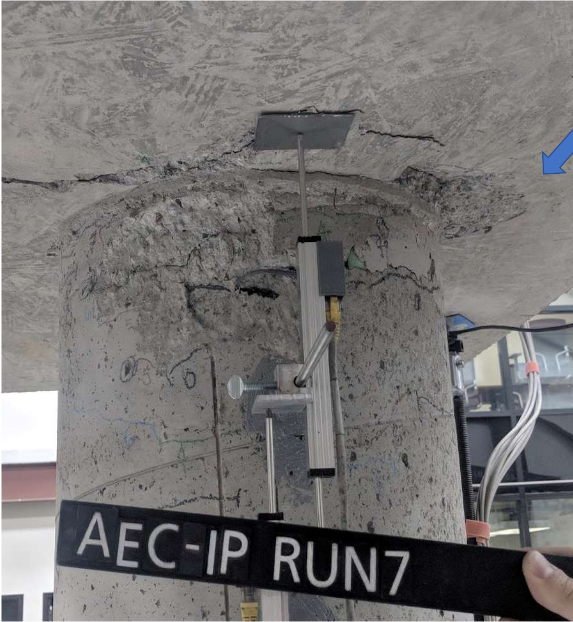
Figure 5.37 Run 7 – Spalling of column and cap beam (CIP – S face)
