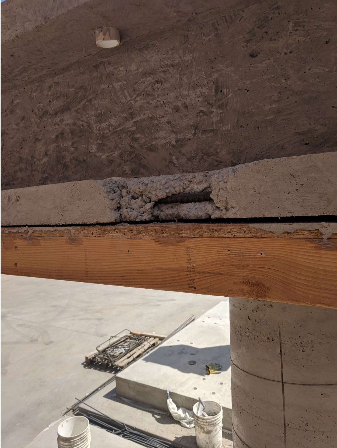
Figure 2.55 Exposed cap beam flange rebar
