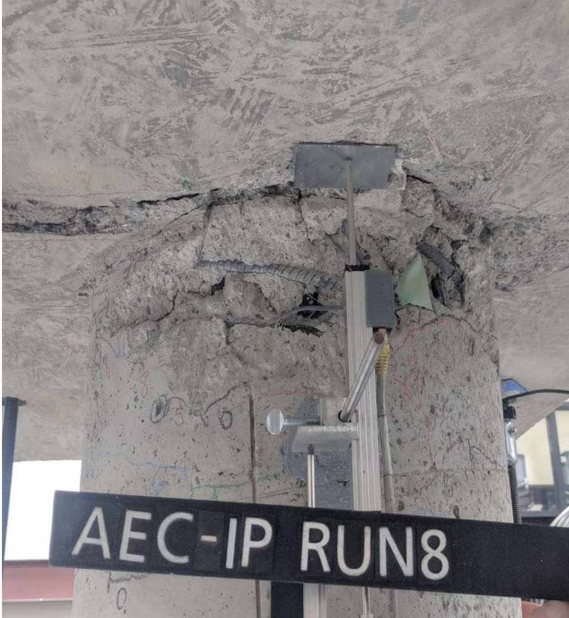
Figure 5.39 Run 8 – Major spalling of column and cap beam and exposure of reinforcement (CIP – S face)
