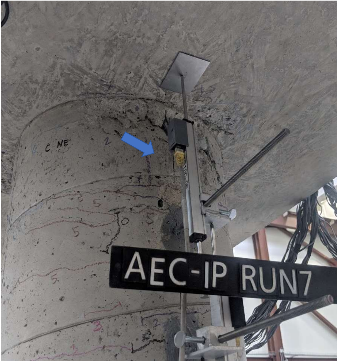
Figure 5.36 Run 7 – Spalling of column and formation of shear crack (CIP – N face)
