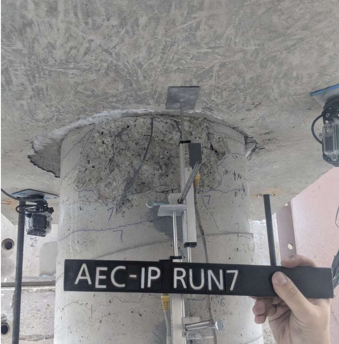
Figure 5.10 Run 7 – Spalling of column (ABC - N face)
