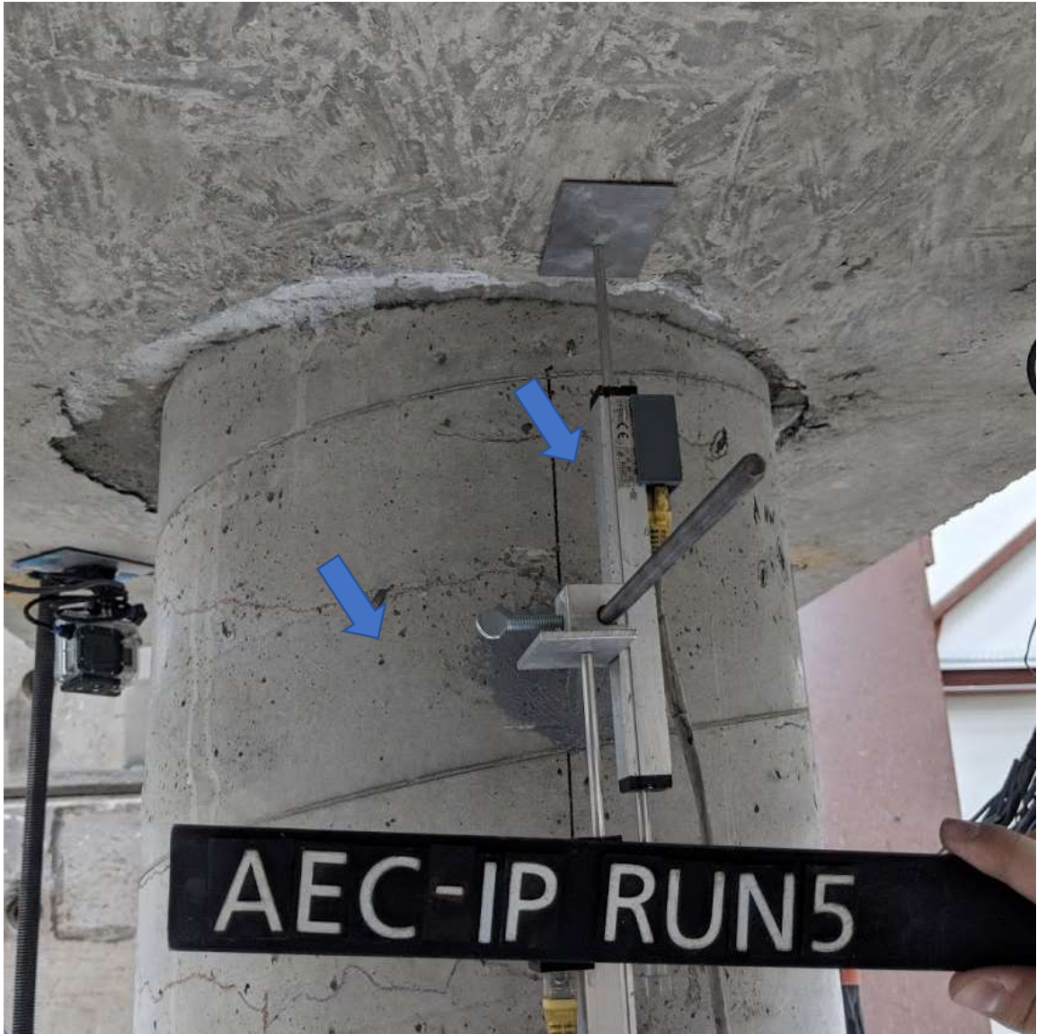
Figure 5.5 Run 5 – Appearance of flexural cracks in plastic hinge (ABC - N face)
