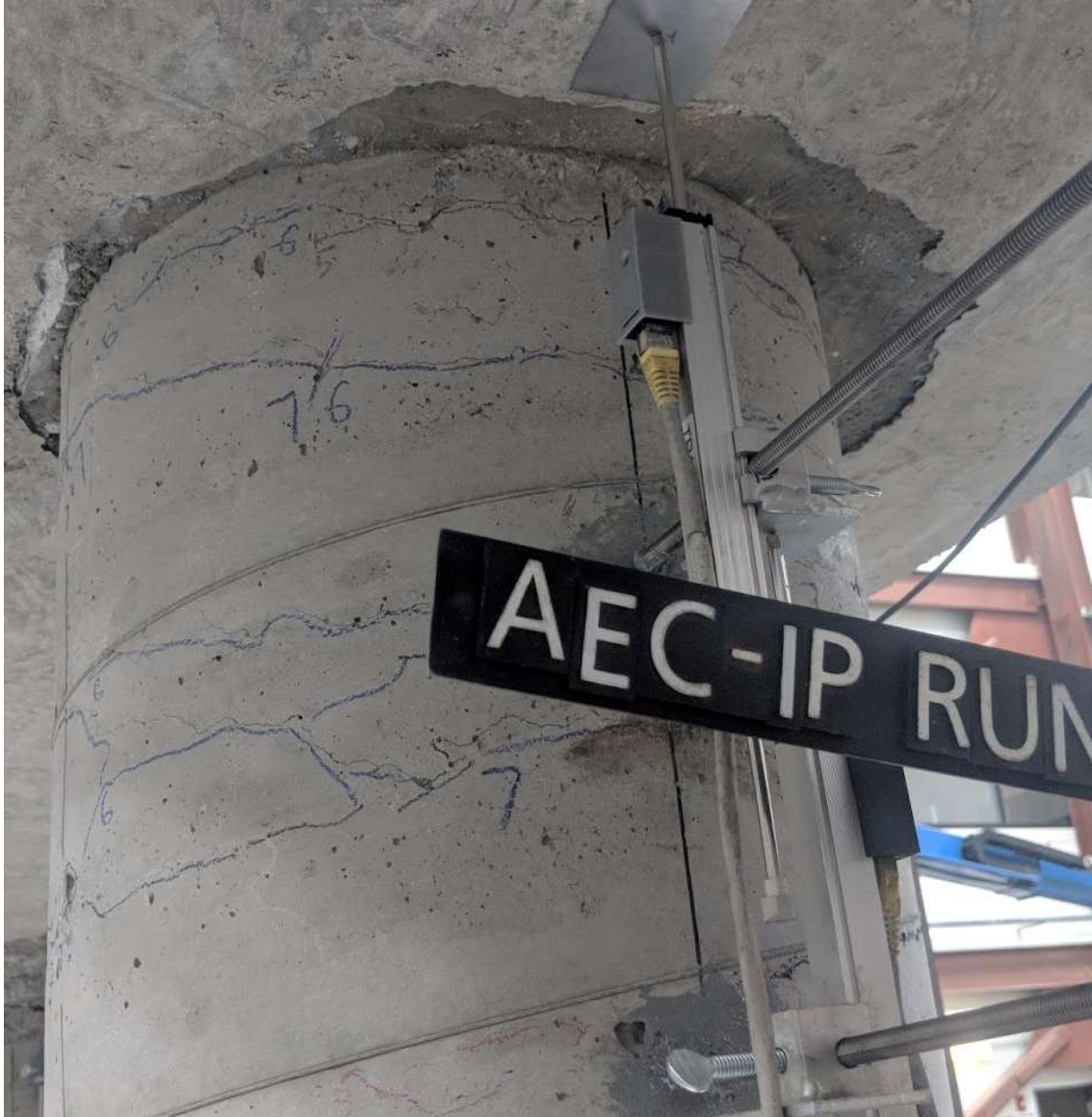
Figure 5.11 Run 7 – Extension and widening of flexural cracks (ABC - S face)
