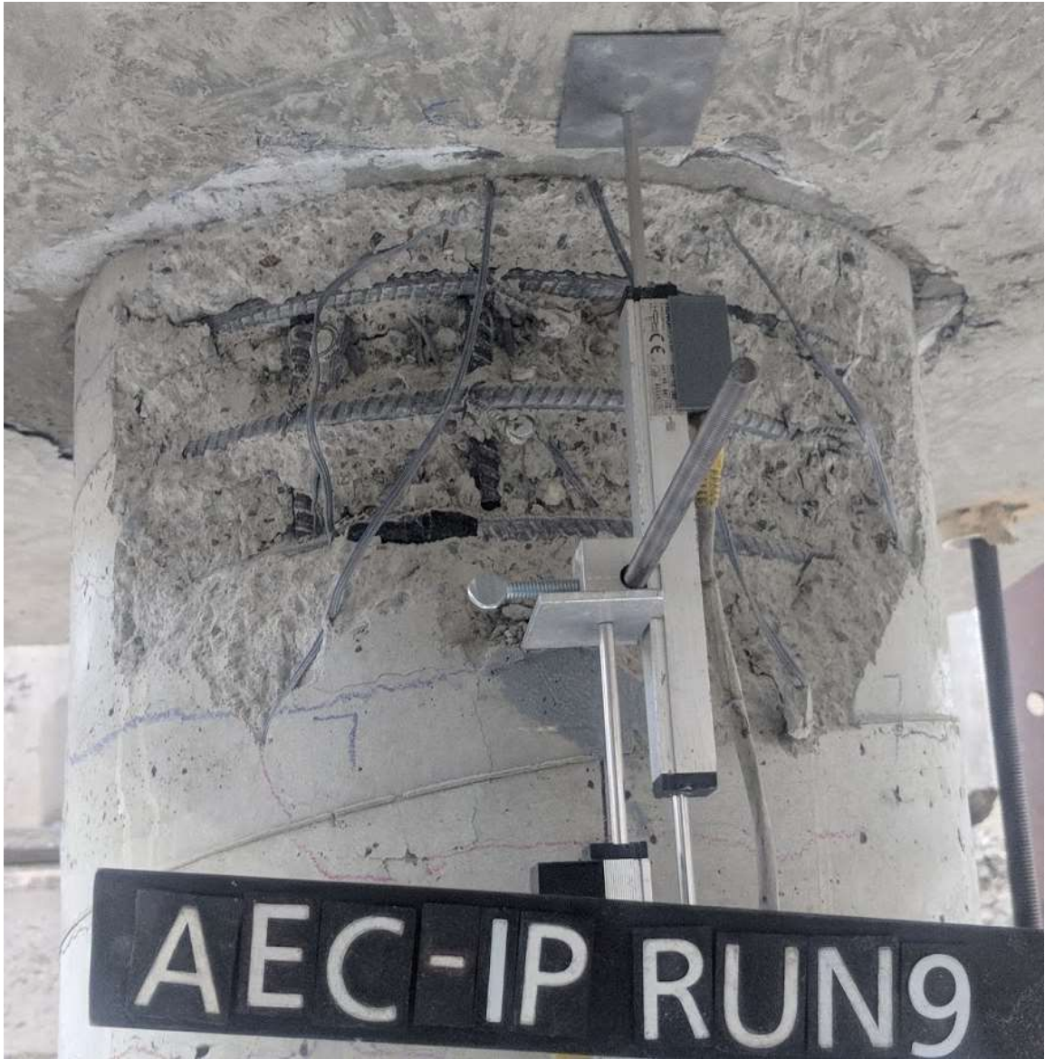
Figure 5.15 Run 9 – Progression of spalling (ABC – N face)
