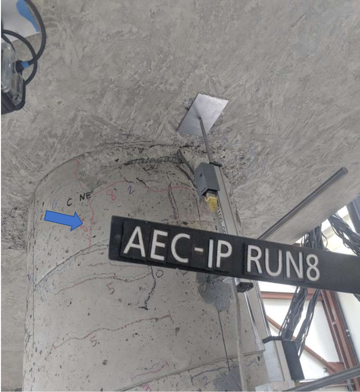
Figure 5.40 Run 8 – Progression of spalling, exposure of reinforcement, and appearance of new shear cracks (CIP – N face)
