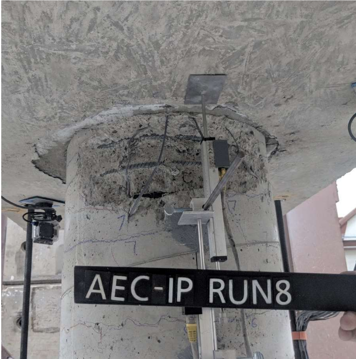
Figure 5.12 Run 8 – Exposure of column reinforcement (ABC - N face)
