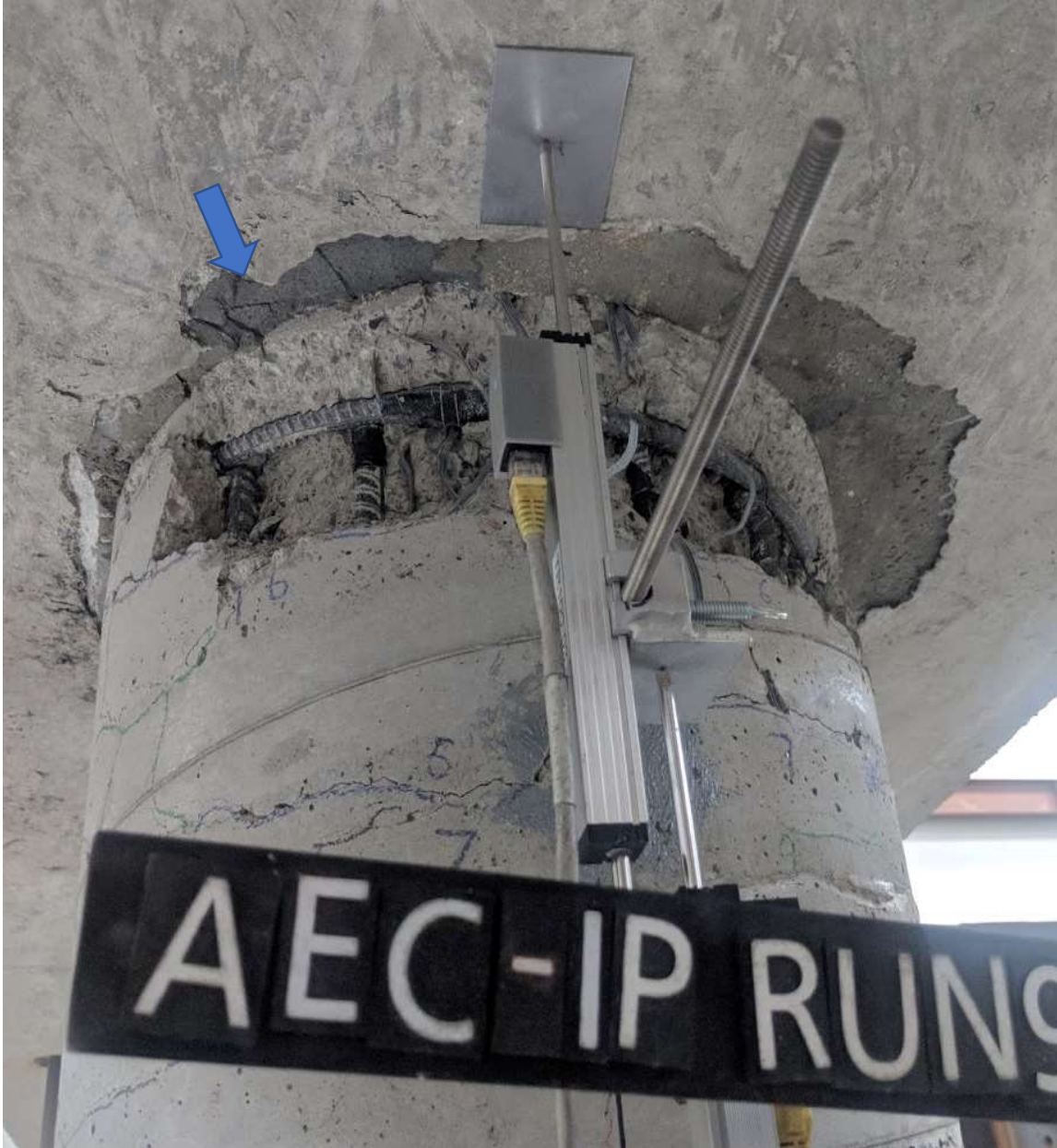
Figure 5.17 Run 9 – Spalling of column, cracking of grout, and exposure of reinforcement (ABC – S face)
