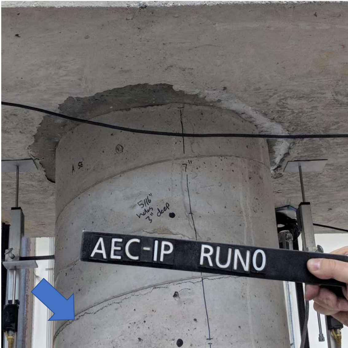
Figure 5.1 Run 0 - Crack along Sonotube form spiral before start of testing (ABC - E face)
