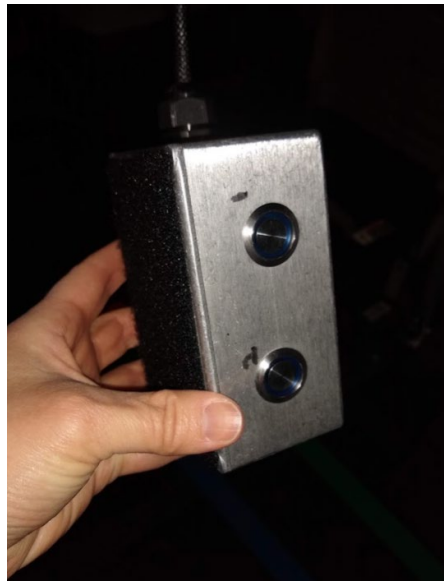
Figure 114. Photo of actuator controls
