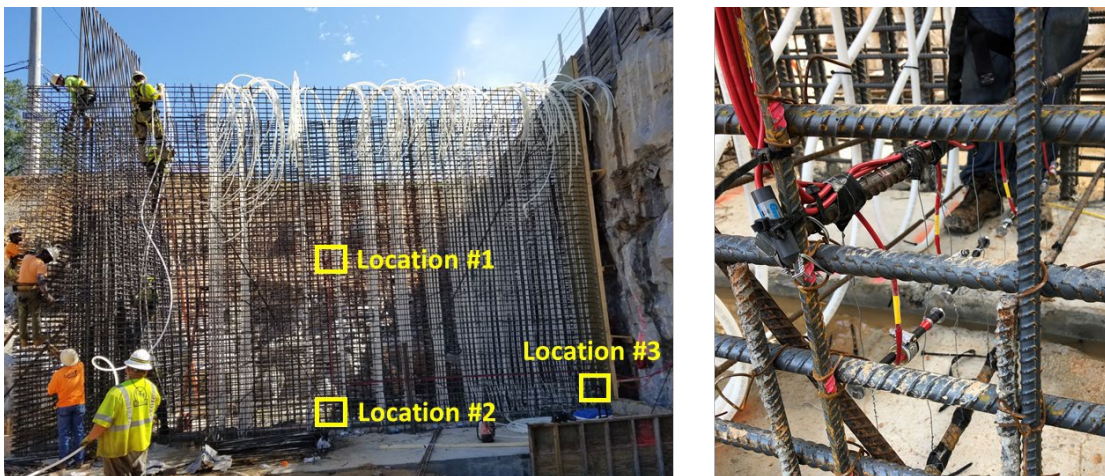
Figure 10. Photos. Sensor locations at the SR-92 abutment.
