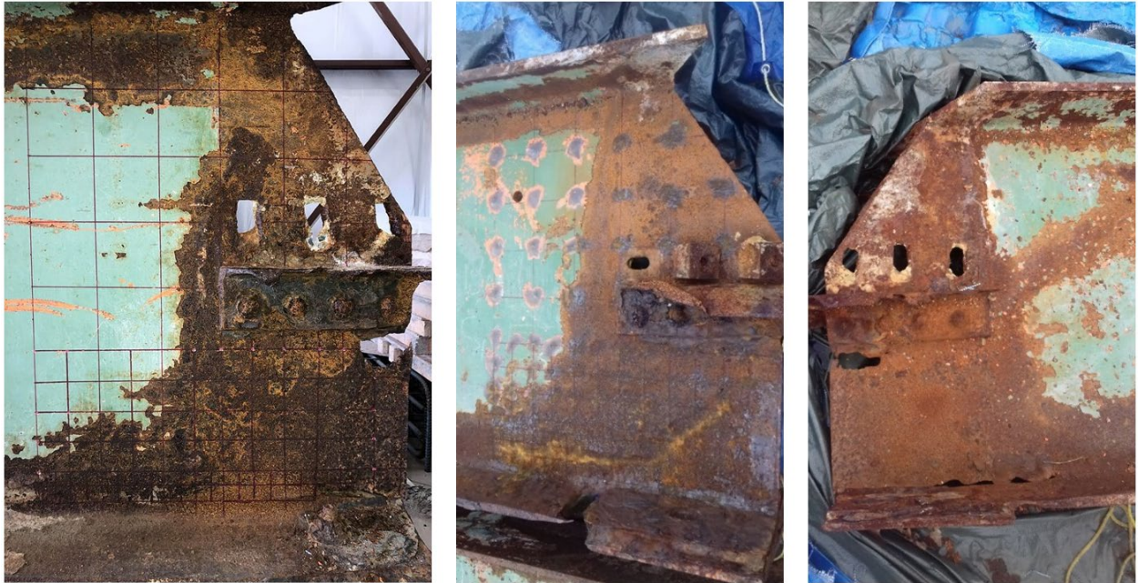
Figure 3.1: Corroded W-shaped bridge beam ends
