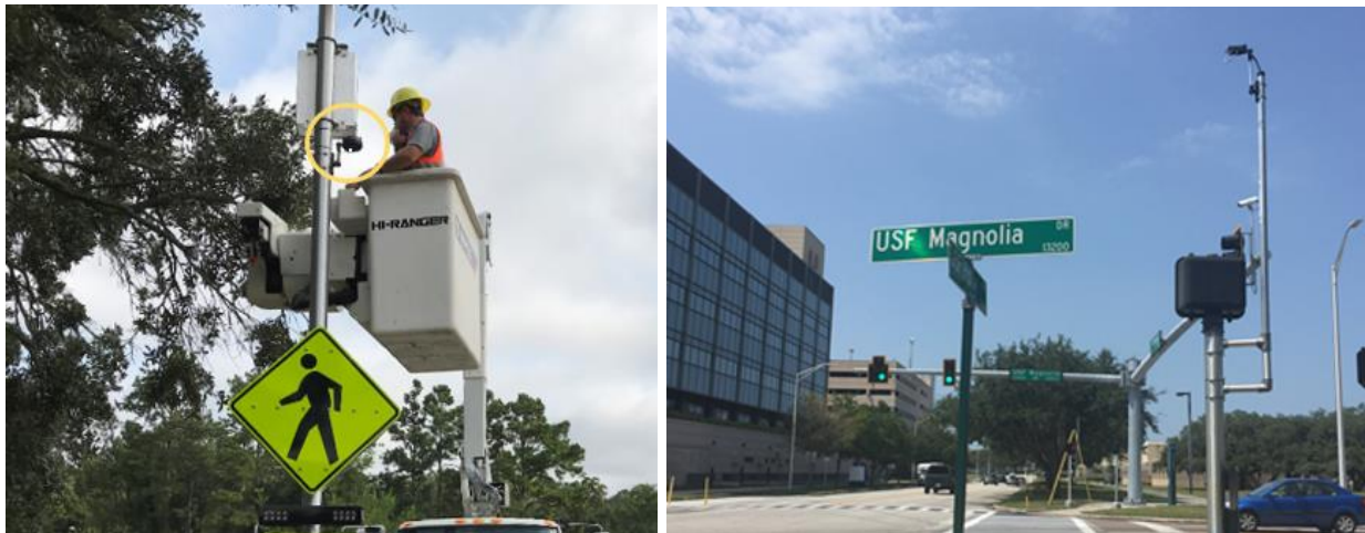
Figure 47. Use of existing pole or extended arm to properly set up automatic pedestrian system
