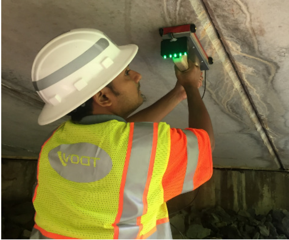
Figure 28. MFLIS Device Scanning Underside of Box Beam. MFLIS = magnetic flux leakage inspection system.
