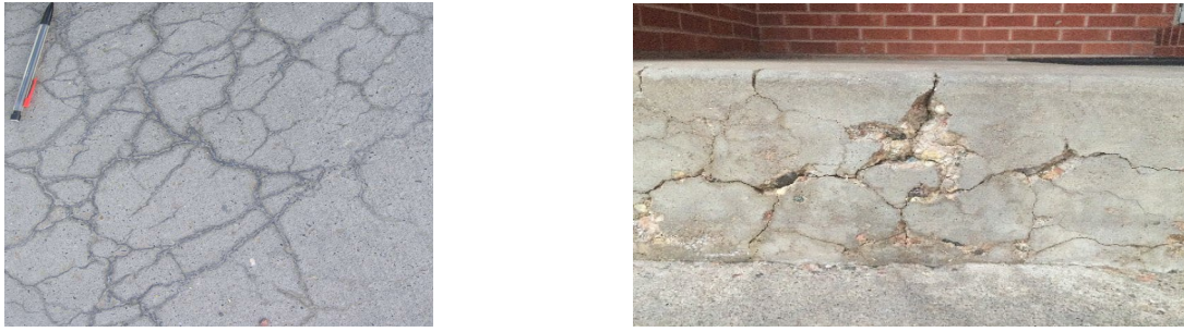
a) Map cracking-Federal Street in Riverton b) pop-outs and map cracking-Cheyenne
