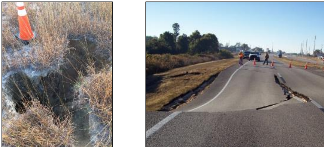
Figure 2-2. (left) Solution sinkhole, (right) cover subsidence sinkhole underneath roadway (Source: FDOT)
