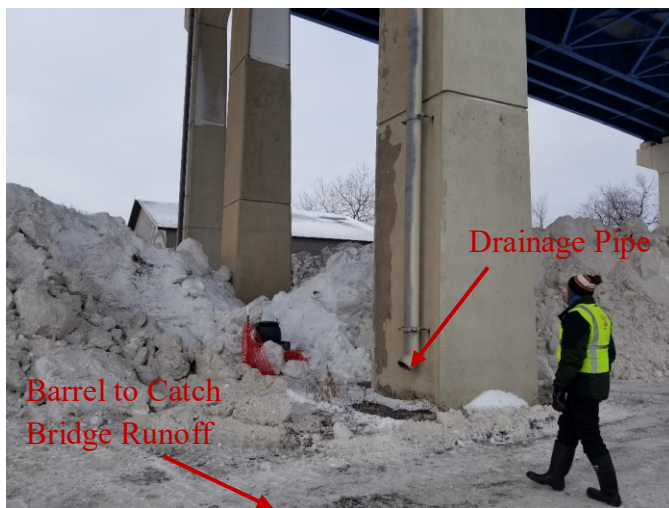
Figure 2.4. Runoff collection for Blatnik Bridge site
