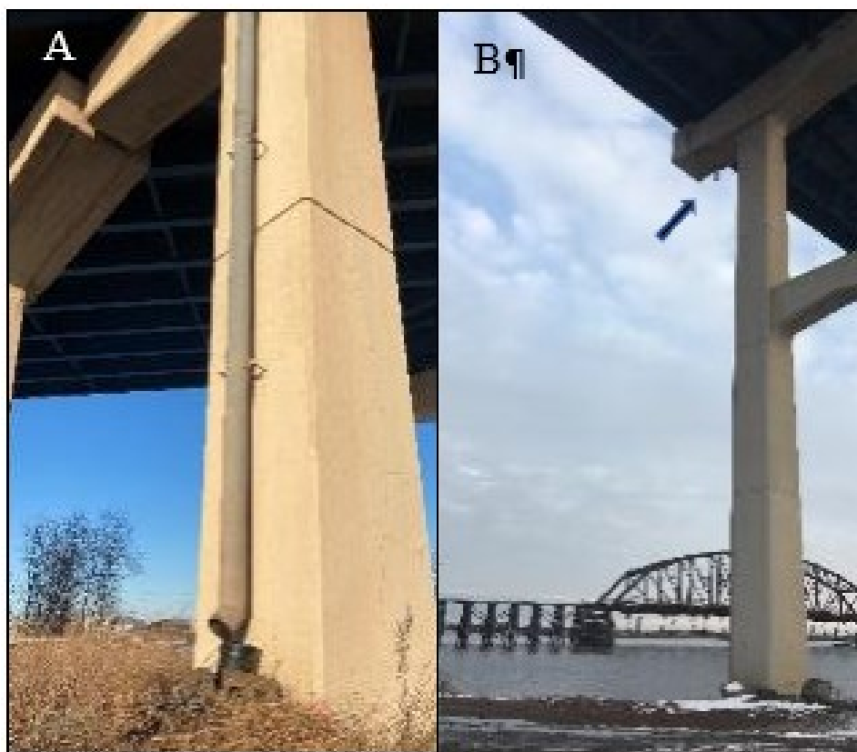
Figure 3.10. (A) BB-KAc-B; with the collection bucket; (B) BB-RP-B, with an arrow pointing to the discharge pipe over the sampling location
