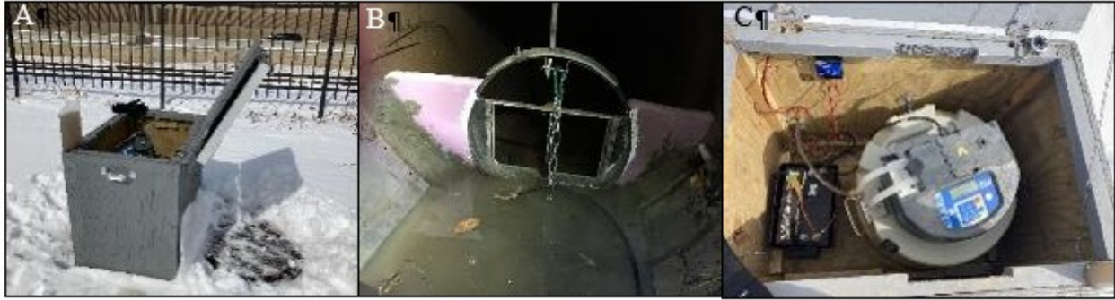
Figure 3.5. Setup at I-35-KAc-A site (A) ISCO sampling unit box and (C) ISCO set up with battery inside the box. The I-35-KAc-A storm drain (B) was sampled with a flow meter and ISCO tubing attached to a spring ring, and a weir to back up flow.
