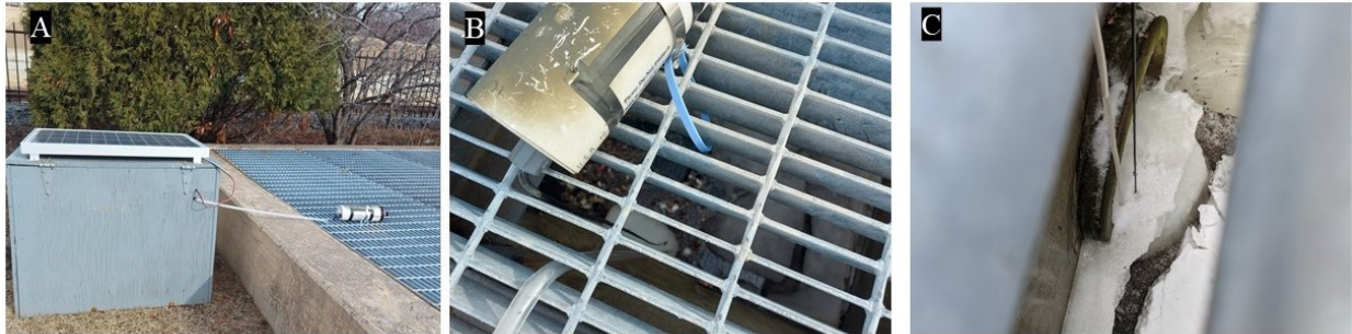
Figure 3.6. (A) ISCO sampling unit box used to collect stormwater from the sedimentation basin, I-35-KAc-B site, (B) ISCO tubing and conductivity/temperature sensor through the metal screen to collect stormwater in the basin, and (C) frozen stormwater in the basin during February-March, 2021
