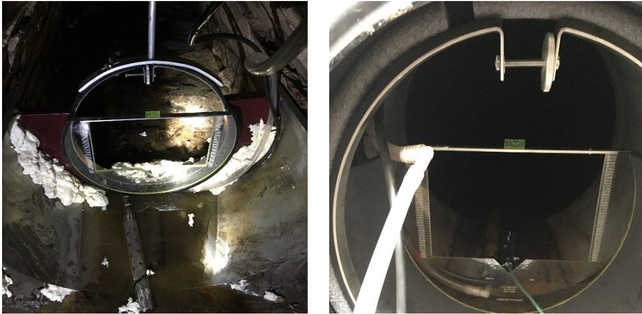
Figure 3.44. Images of weir modification with cements and foam to capture low flow of snowmelt runoff
