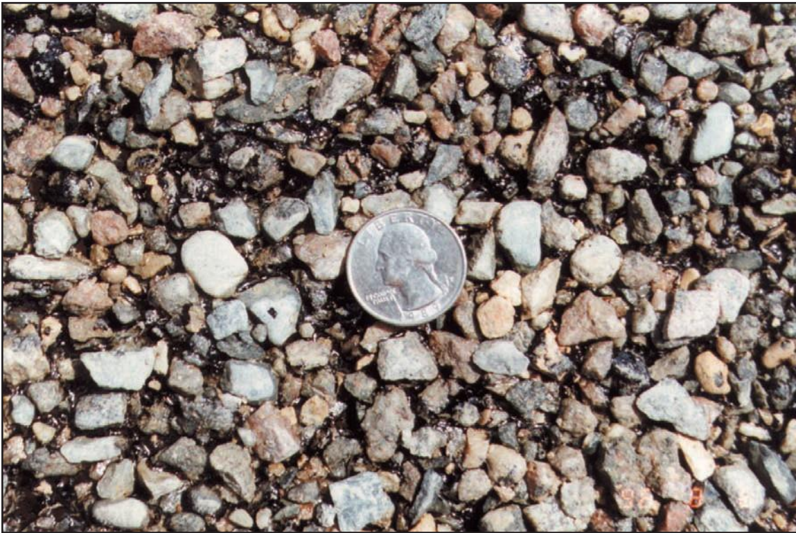
Figure 3.7.3. Not enough binder (binder is too low)
