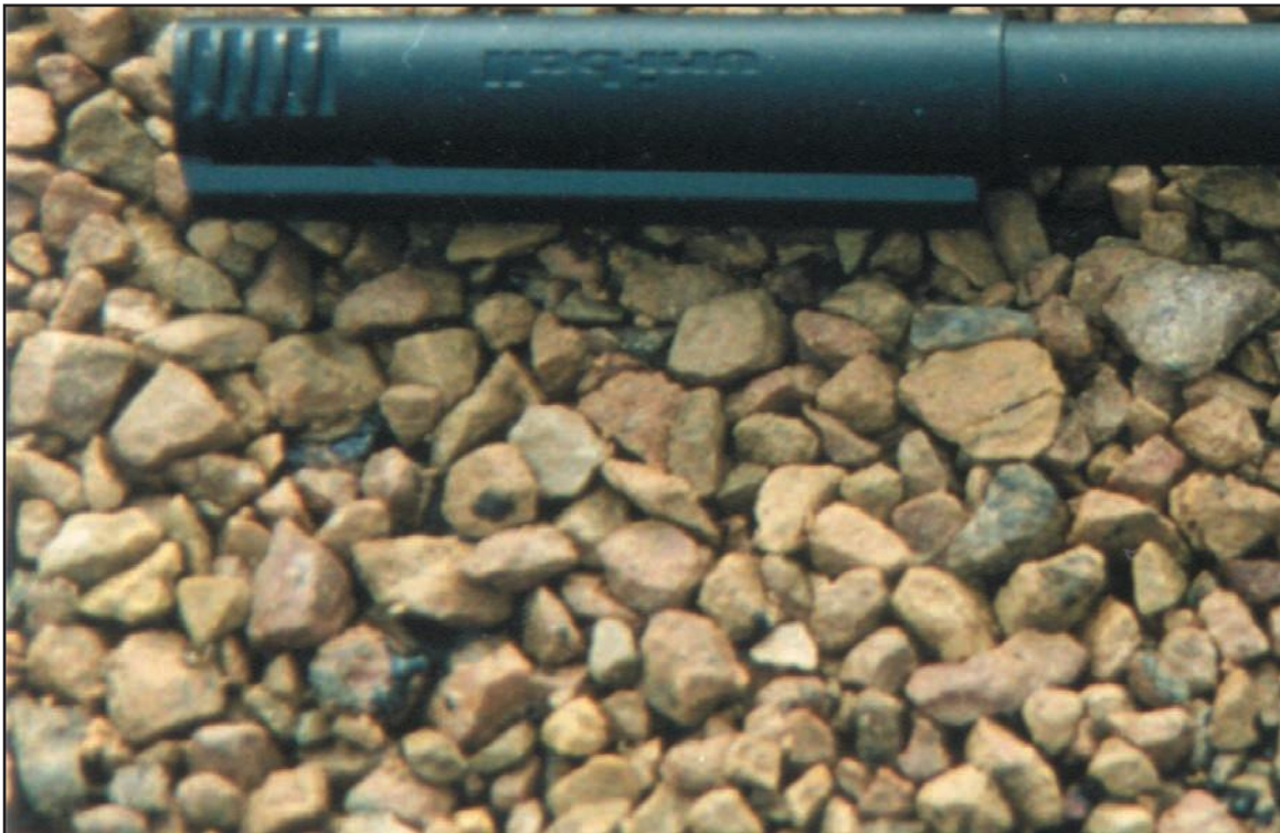
Figure 3.7.2. Too much aggregate (no binder is visible)
