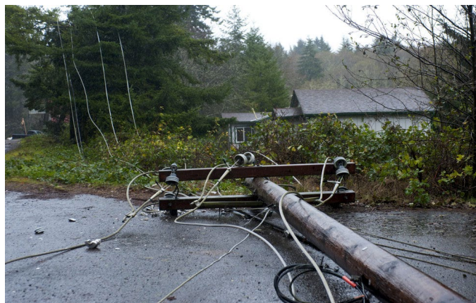
Figure 29. Photo. Fallen power lines – Library sample image. (34)
