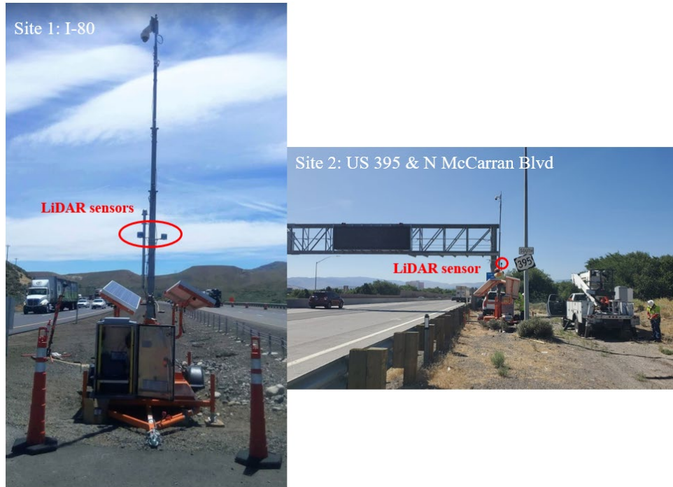
Figure 4-4 ITS trailer equipped with two LiDAR sensors
