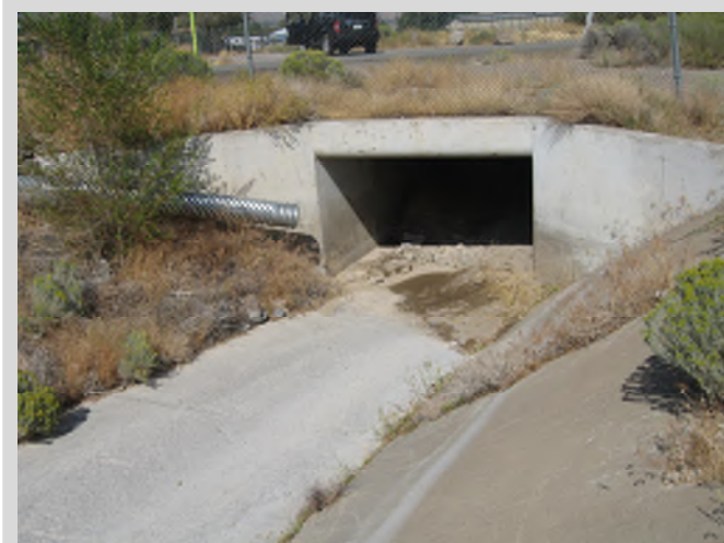
12'x5' concrete box culvert at Bailey Canyon Creek crossing under Kivett Lane
