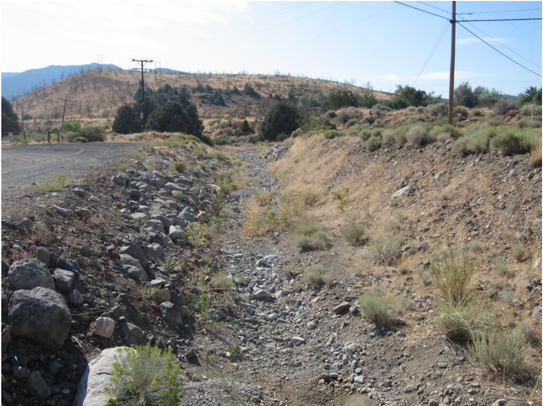
Photo: Bailey Canyon Creek Culvert Crossing at Toll Road. Looking upstream (southeast) at upstream channel. (Photo Date: 9/16/2011)
