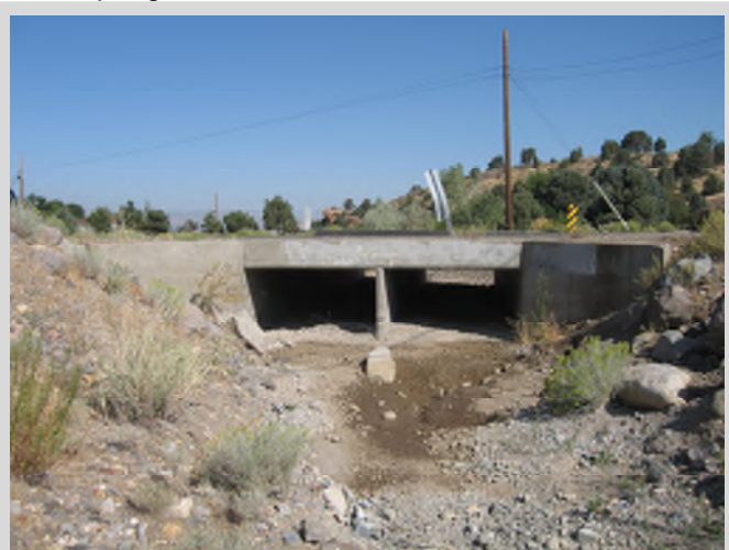
Dual 8'x5' concrete box culverts at Bailey Canyon Creek crossing under Toll Road near Ravazza Road
