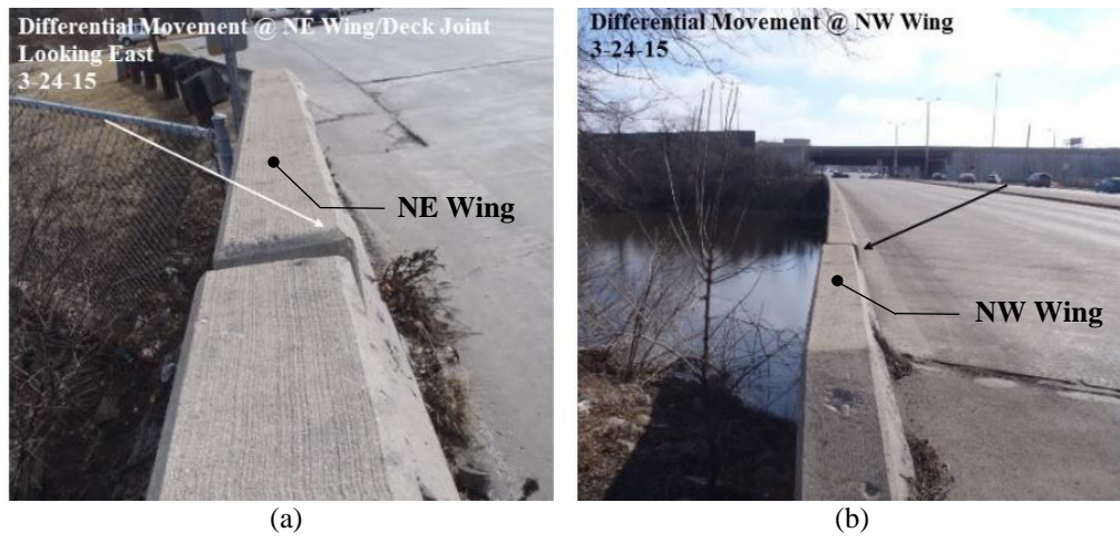
Figure 2.5. Misalignment of wingwall and bridge parapet wall at (a) acute, and (b) obtuse corners. [1]
