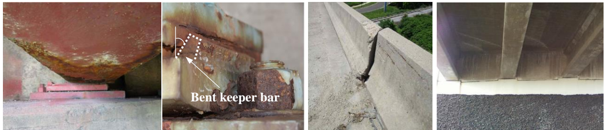
Figure A. Misaligned girder (left), bent keeper bar (middle, left) misaligned parapet wall and closed expansion joint (middle, right), diagonal acute corner deck cracks (right). [1]
