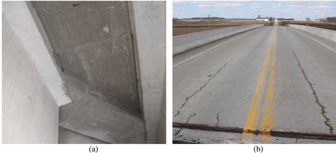
Figure 3.1. (a) Lack of cracking on deck bottom surface for 52° skew, and (b) longitudinal cracks for 0° skew near the abutment.
