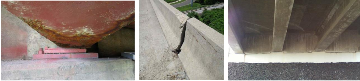
Figure 1.2. Misaligned girder (left), misaligned parapet wall and closed expansion joint (middle) of B-13-228, diagonal acute corner deck cracks (right) of B-09-212. [1]
