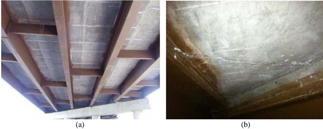
Figure 3.9. Deck bottom face: (a) transverse cracking on west span, and (b) typical acute corner cracking at bridge ends of the load tested steel bridge.
