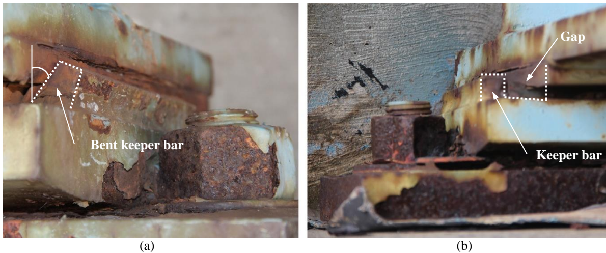
Figure 3.5. (a) Bent interior keeper bar and (b) gap between bearing and exterior keeper bar of obtuse corner bearing at north bridge end for 30° skew.
