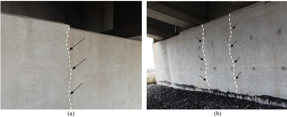
Figure 3.6. Vertical abutment cracks for bridges with (a) 52° skew, and (b) 0° skew.
