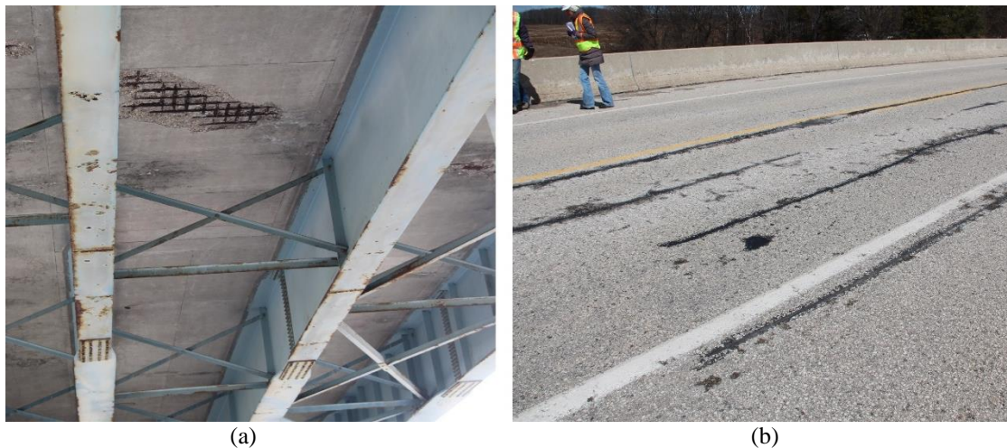
Figure 3.2. (a) Concrete spalling on deck bottom surface for 30° skew, and (b) longitudinal sealed cracks on deck top surface for 3° skew.
