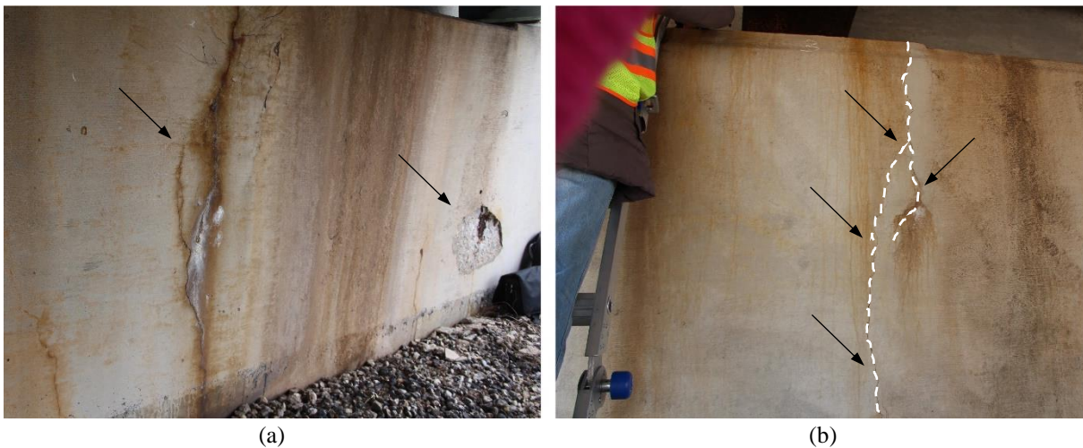
Figure 3.7. Vertical cracks on the abutments of bridges with (a) 30° skew, and (b) 3° skew.
