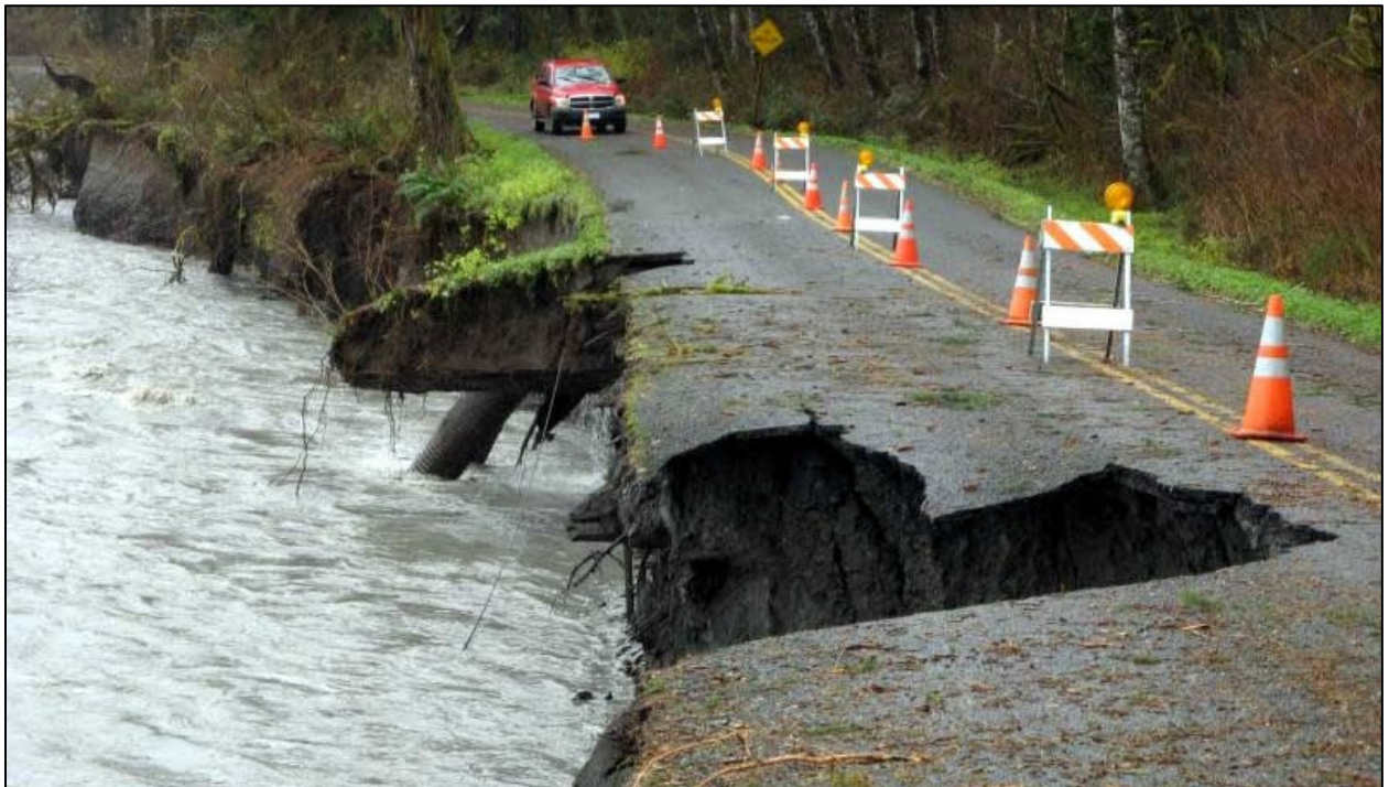
Figure 73. Embankment and roadway erosion along banks of Hoh River (NPS 2021).
