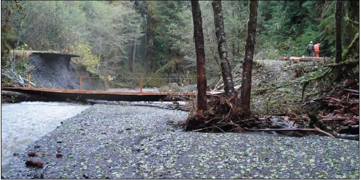
Figure 48. Washout of earlier bridge crossings (NPS 2021).
