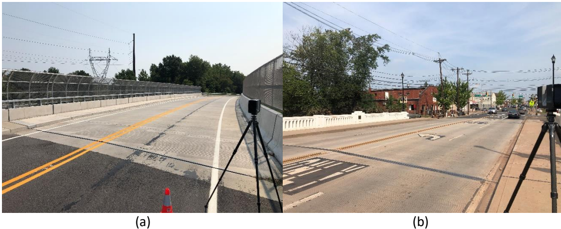
Figure 13. Typical location of scanner: (a) Scanner located on deck's shoulder; (b) Scanner located on sidewalk.
