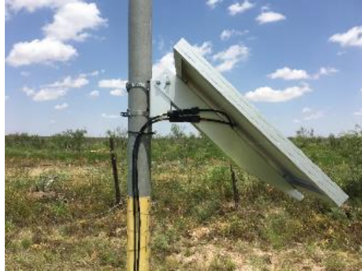
Figure 50. Solar Panel Mounted on a Pole.
