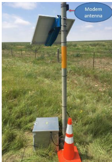
Figure 59. Attached Modem Antenna.
