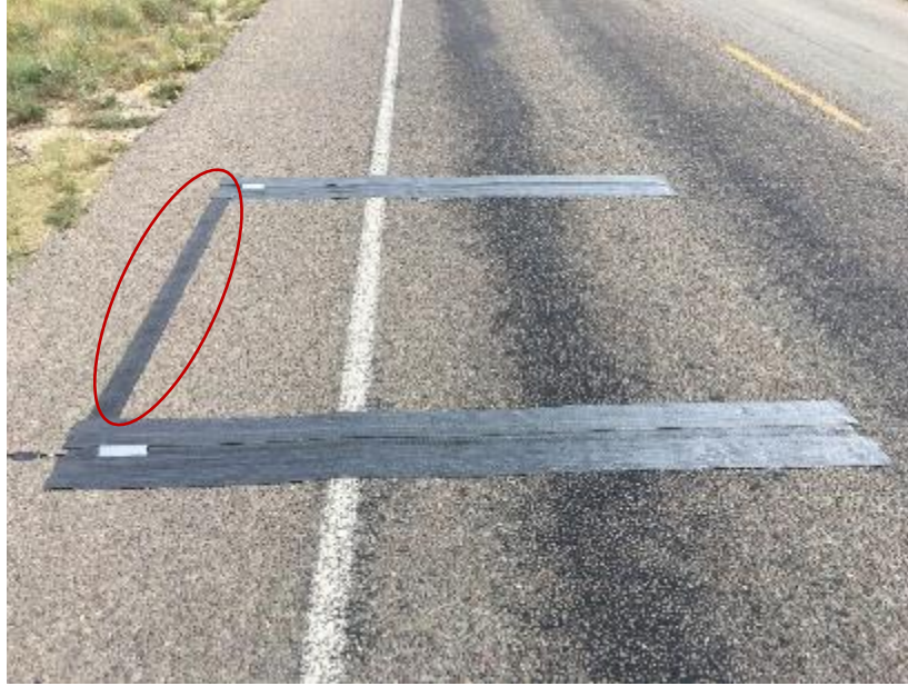
Figure 43. 4-Inch Road Tape Applied on the Shoulder to Cover the Sensor Cables.
