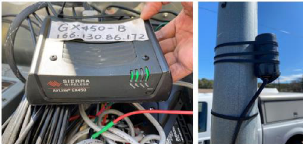
Figure I-5. Modem Communication System for the Portable WIM.
