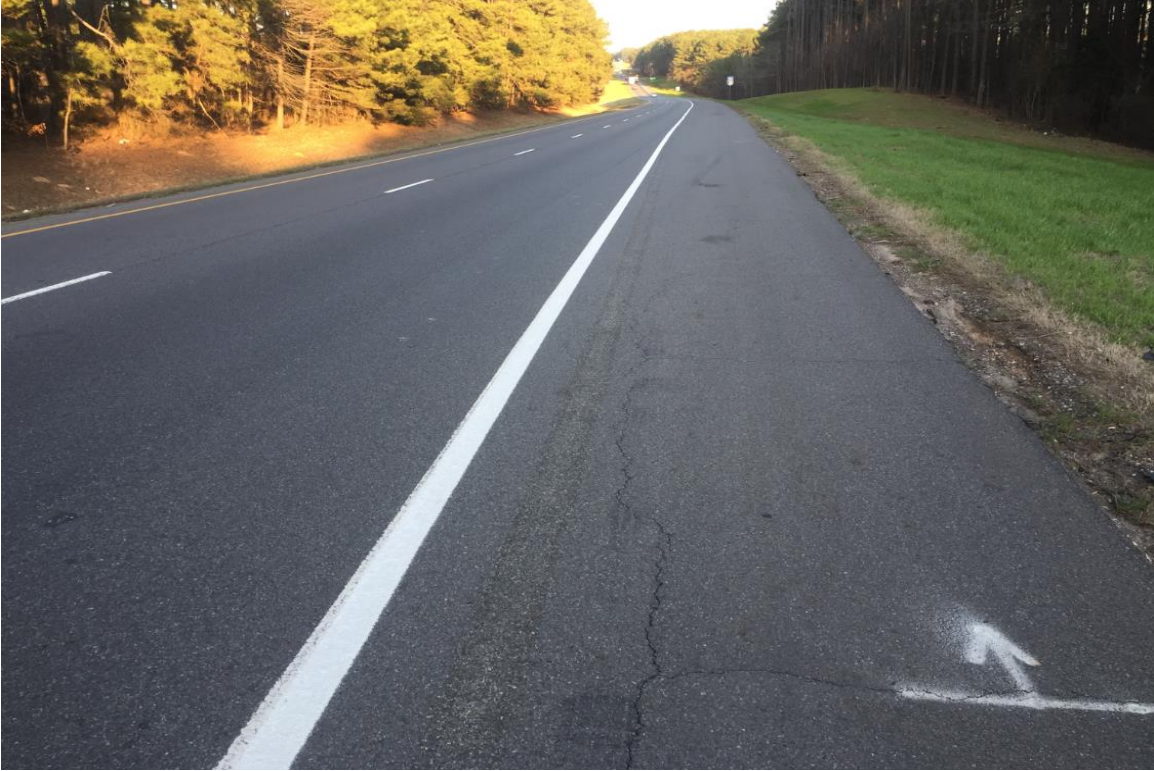
Figure 3-25. IH 20 Pavement Surface Condition in March 2021.
