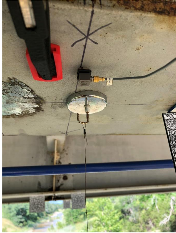
(b) Example of Installed Accelerometer
