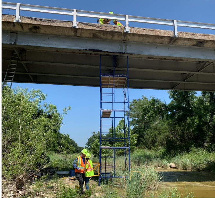
(a) Instrumentation of Bridge SC-12
