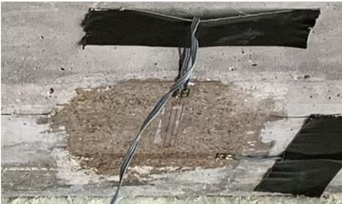
Figure 9.4. Close-Up of Strain Gauge Installation
