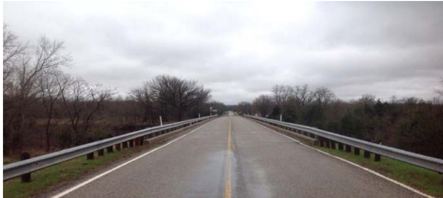
(b) Roadway View—No Cross-Section plans available for the steel continuous section of this bridge
