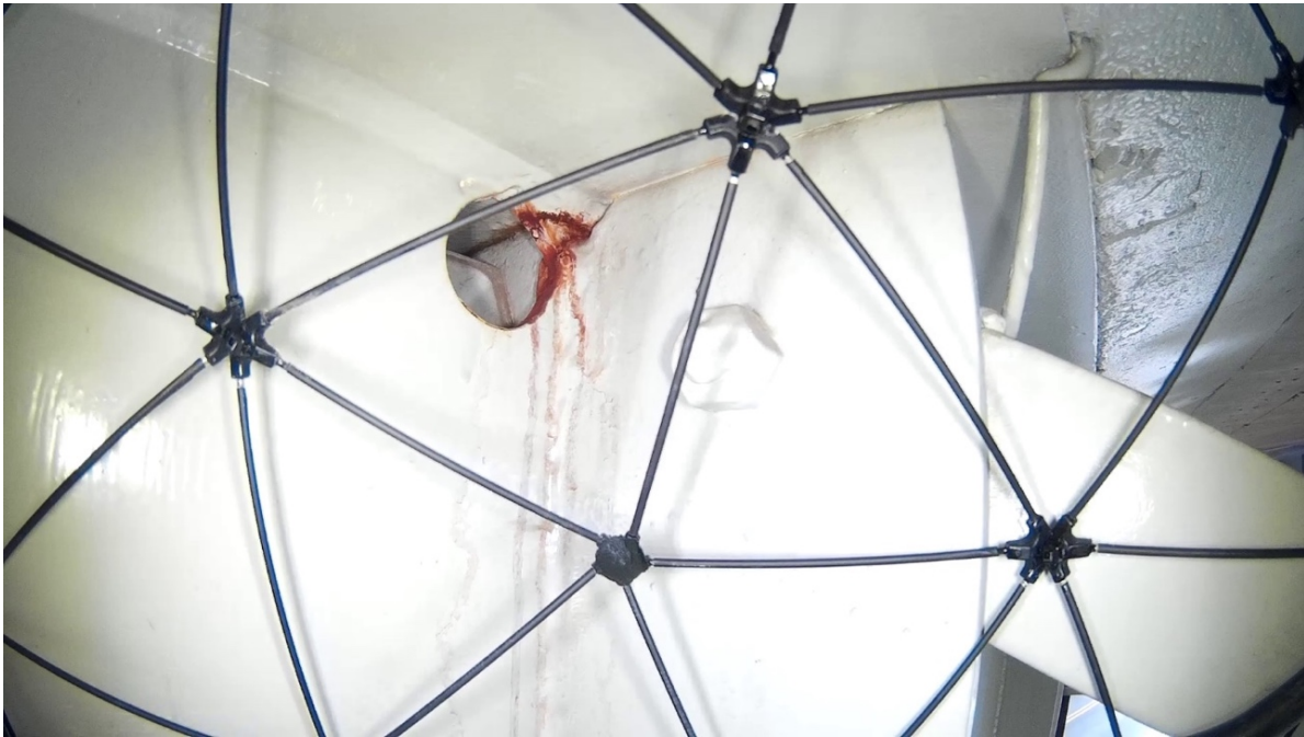
Figure 146: Inspection of Stress Crack
