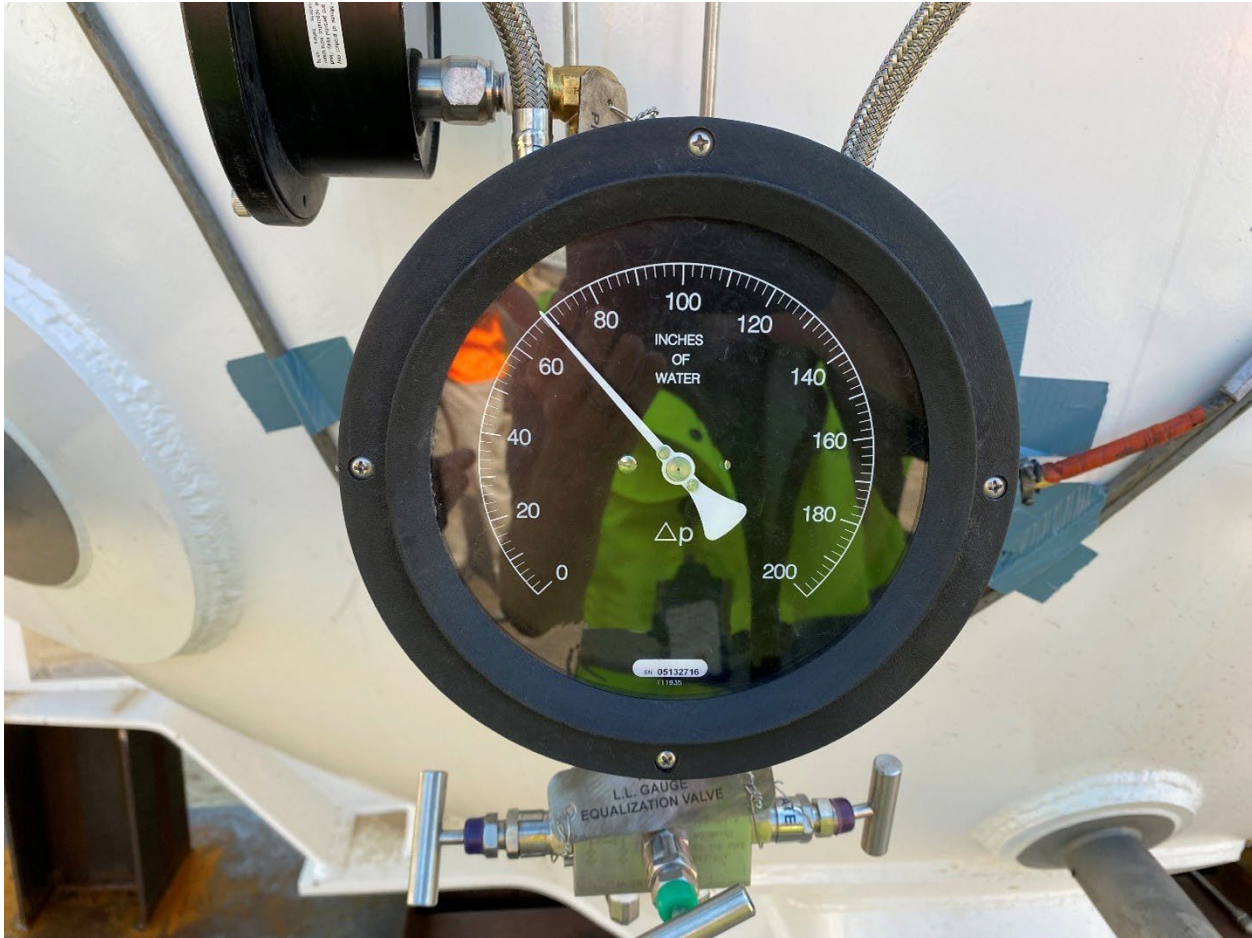
Figure 42. Static Head Pressure Gauge, Day Before Test
