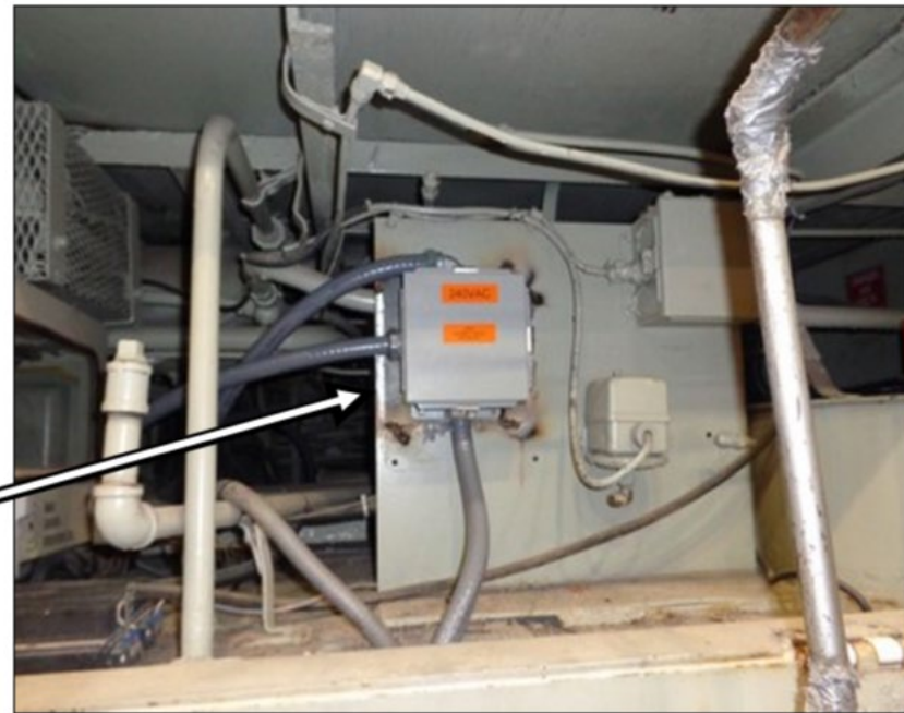
Figure 7 – EPSS locomotive junction box
