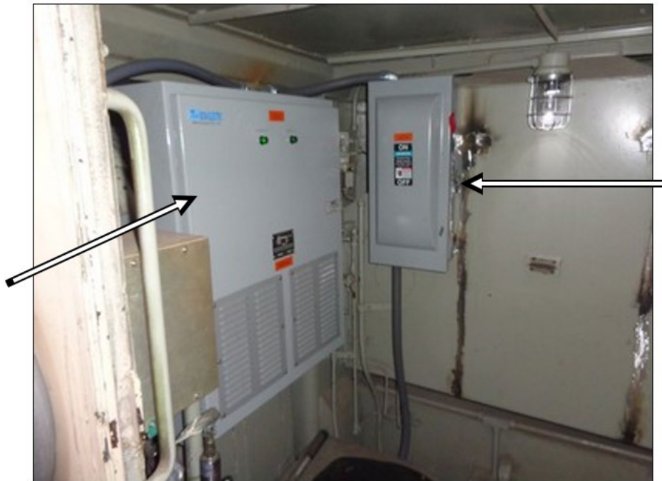
Figure 5 – EPSS inverter (left) and supply disconnect
