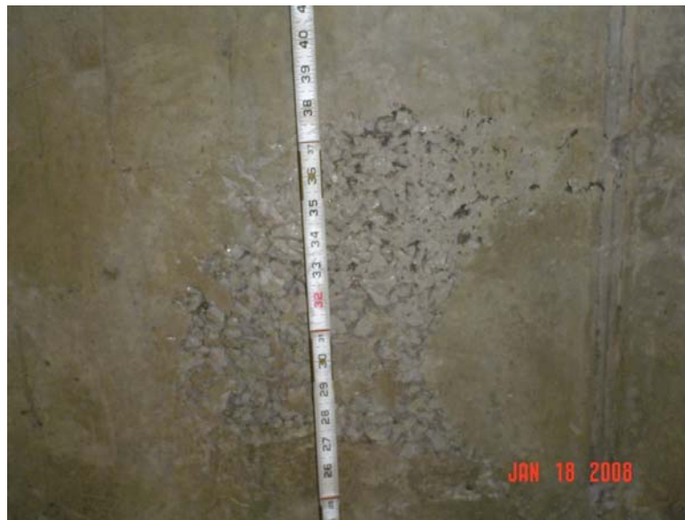
Figure 8.9: Honeycombing in the Wall of Structure #52-489-339
