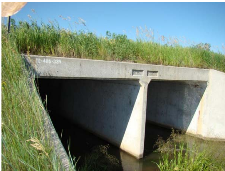
Figure 8.14: Structure #52-489-339 after One Winter in Service
