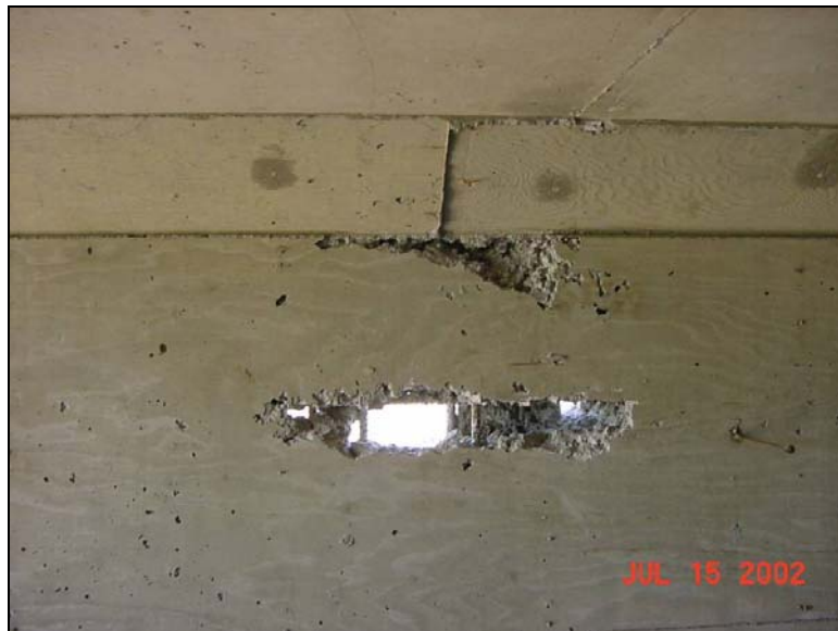
Figure 2.1: Concrete Void in the Wall of a Cast-In-Place Box Culvert (Courtesy SDDOT)
