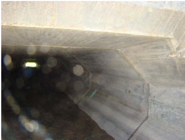
Figure 8.13: Structure #52-485-337 after One Winter in Service
