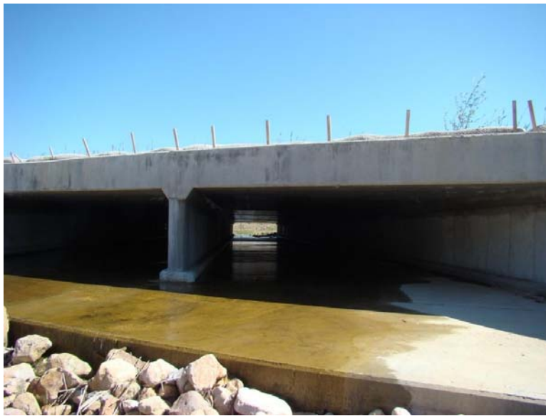
Figure 8.16: Structure #52-462-326 after One Winter in Service
