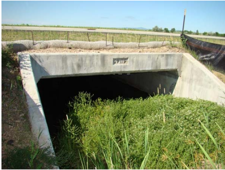
Figure 8.15: Structure #52-472-331 after One Winter in Service
