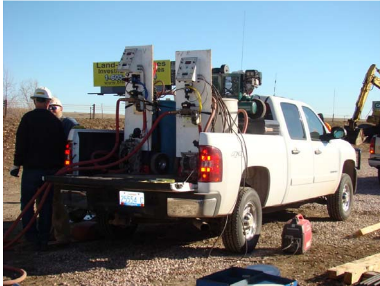
Figure 8.7: Superplasticizer and VMA Pump System
